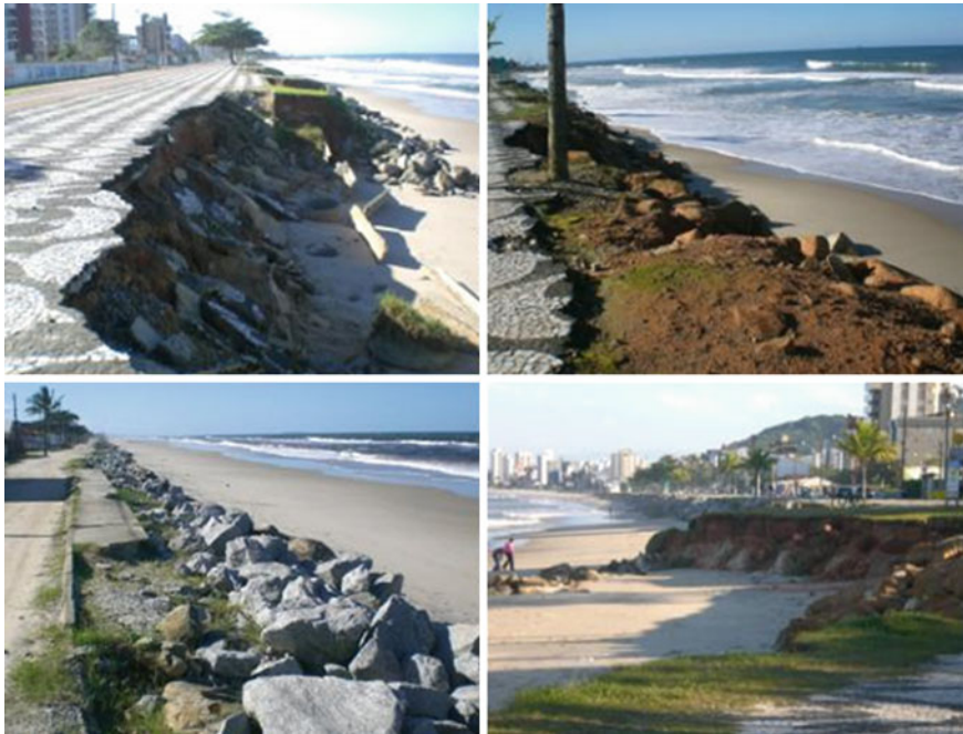
Fig. 12.3 Impacts of shoreline erosion in Matinhos District in the coast of Paraná State, Brazil in 2007. Source Goncalves (2010)
