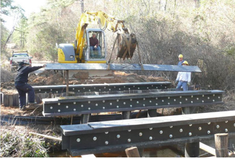
Fig. 10.8 Installation of one inch steel sill plate on pile caps with pre-drilled holes to serve as a template for girder installation
