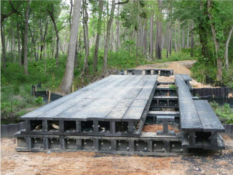
Fig. 10.22 Sub-structure of T85-19 showing the 42 foot girders staggered at one-third of the girder length to achieve a bridge span of 56 ft
