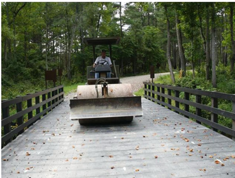
Fig. 10.27 A successful crossing of a 30 ton steam roller over bridge T85-19 after repair of the decking
