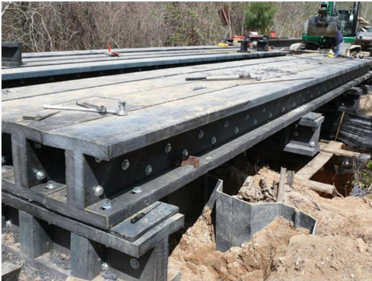
Fig. 10.21 Girder and pile cap I-beam (18 in x 18 in x 42 ft) molded as two T-beams that are glued and bolted together
