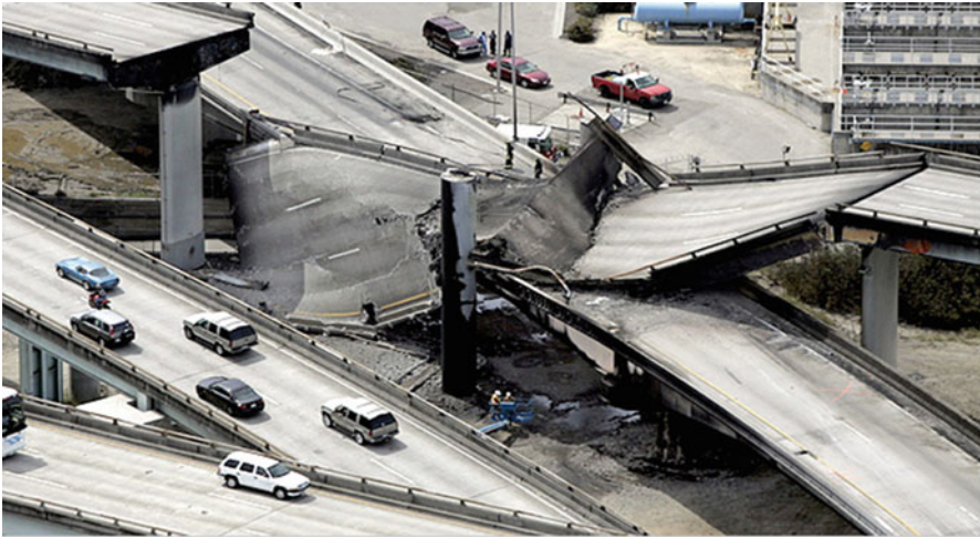
Picture 6.1 I-580/I-880 collapse caused by a tanker truck fire on April 29, 2007 ( The San Francisco Chronicle website, accessed November 5, 2009)
