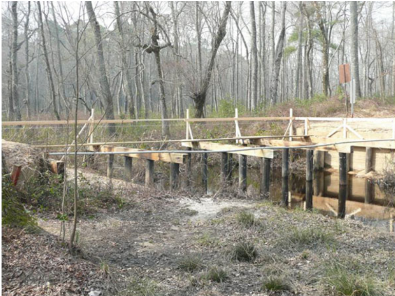
Fig. 10.6 Three rows of five RTCL pilings each on T85-18 with wooden framework for construction purposes
