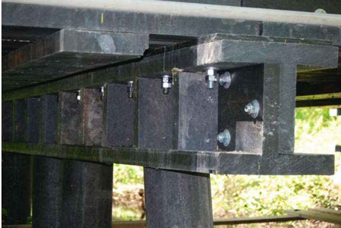
Fig. 10.20 3 by 12 in. stiffeners installed every 18 in. in the web of the pile cap I-beam
