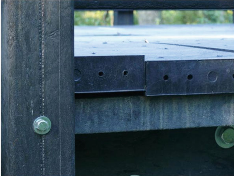
Fig. 10.26 A deck board dislodged 0.5 in above the deck surface on bridge T85-19 after the bridge was traversed by a 30 ton steam roller
