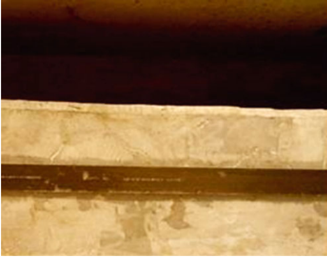
Fig. 11.7 Cracking observed during inspection, looking at the bottom of the beam
