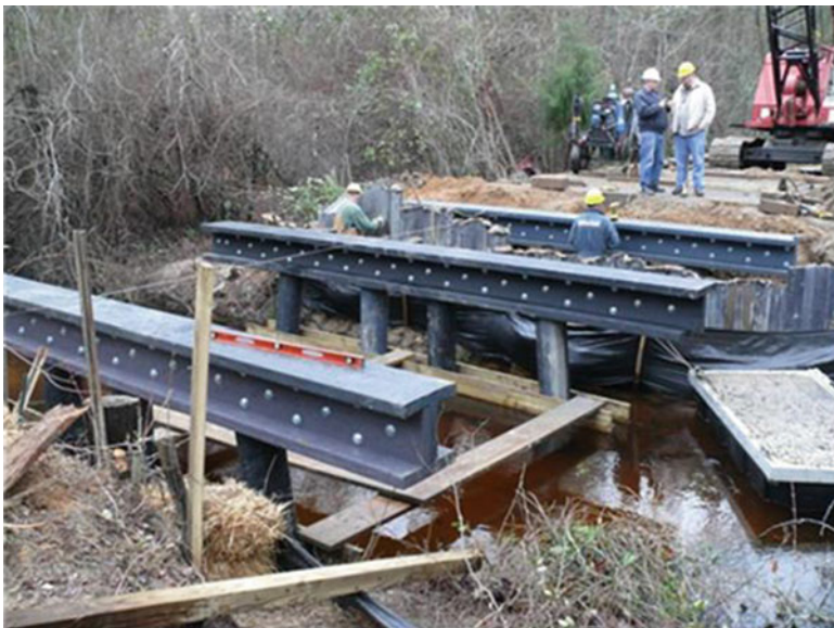
Fig. 10.7 Pile caps in place and pinned on three row of pilings on T85-18
