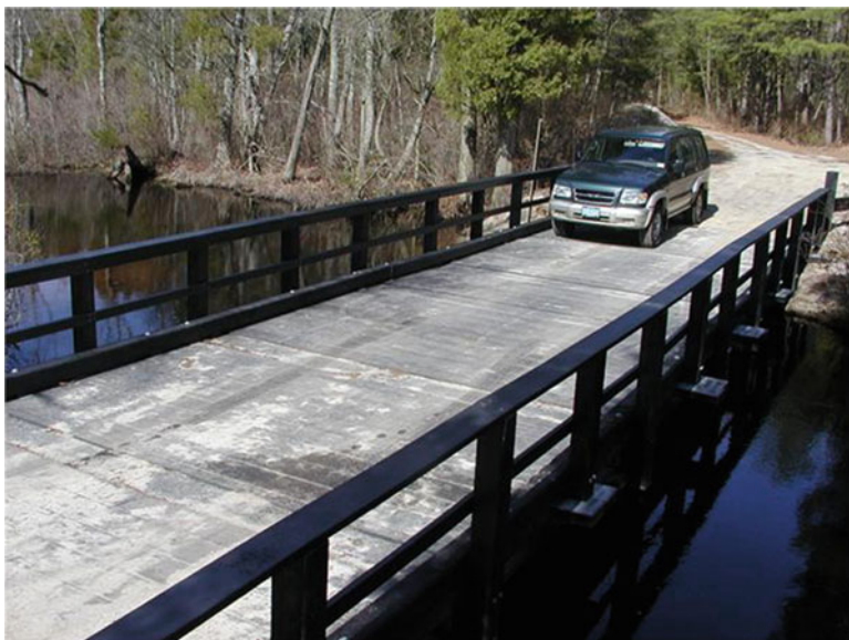
Fig. 10.4 Vehicular bridge in Wharton State Forest, NJ, built in 2002 with an I-beam sub-structure and a maximum load capacity of 36 tons
