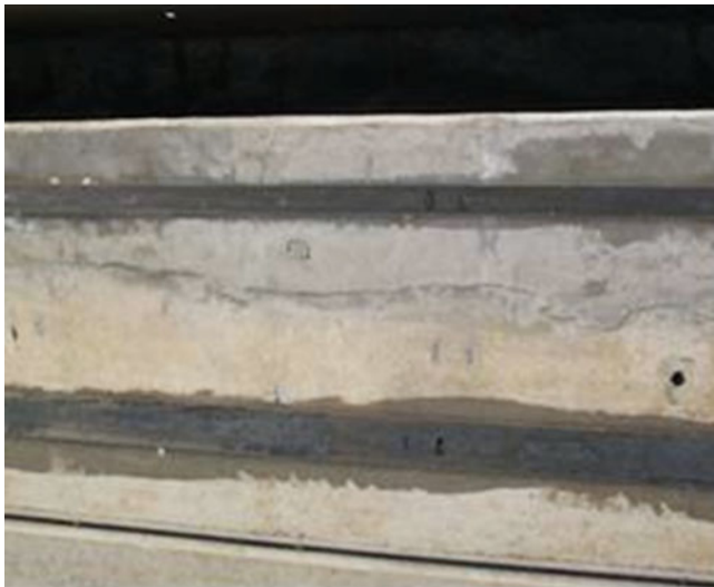
Fig. 11.9 Cracking observed at interface of patch and concrete beam
