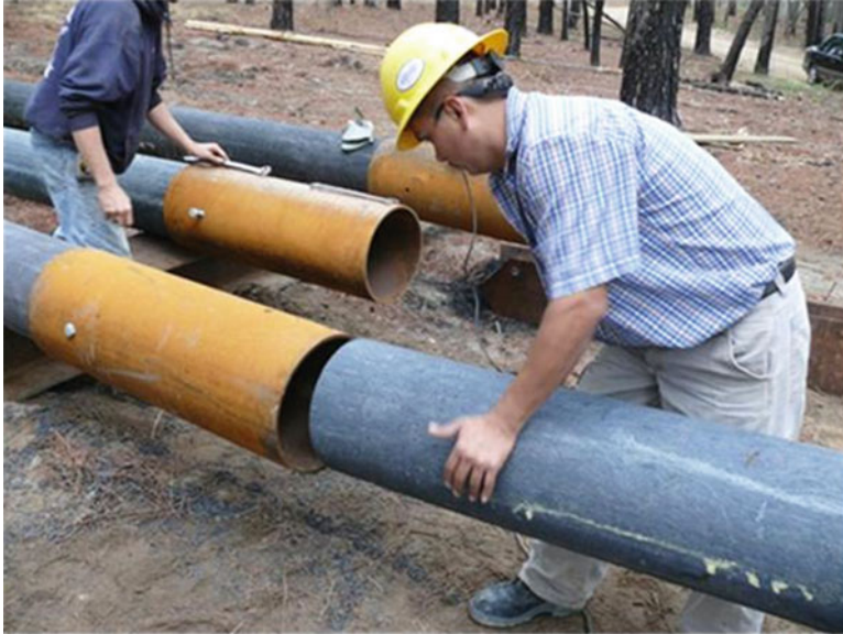
Fig. 10.17 Spliced pilings to achieve the depths needed for 37.5 ton refusal on bridge T85-19
