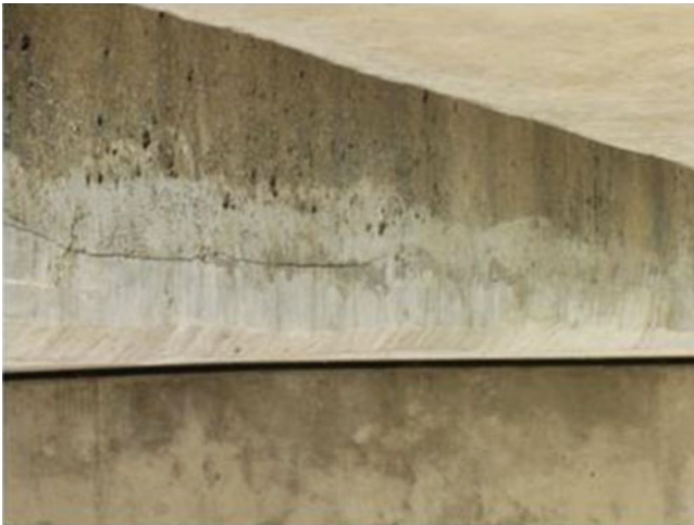
Fig. 11.8 Cracking observed at interface of patch and concrete beam
