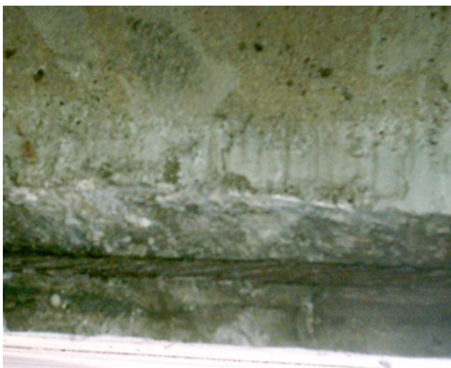
Fig. 11.6 Removed section of unsound patching material, looking at the side of the beam
