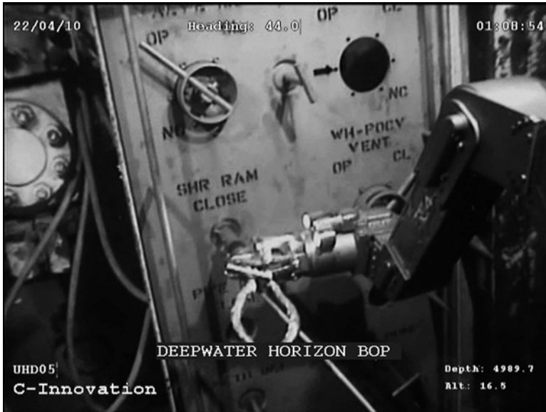
Fig. 7.9 A robotic arm of a Remotely Operated Vehicle (ROV) attempts to activate the Deepwater Horizon Blowout Preventer, on April 22, 2010, 01:08:54 hours, about 2 days after the blowout. When the switch was activated, the BOP stack shook, indicating that the compressed nitrogen cylinders discharged, and the shear ram might have closed. The ram might not have activated automatically upon disconnect from the sinking Deepwater Horizon. For the initial erosion around the ram to occur, the ram must have been partially closed from the beginning
