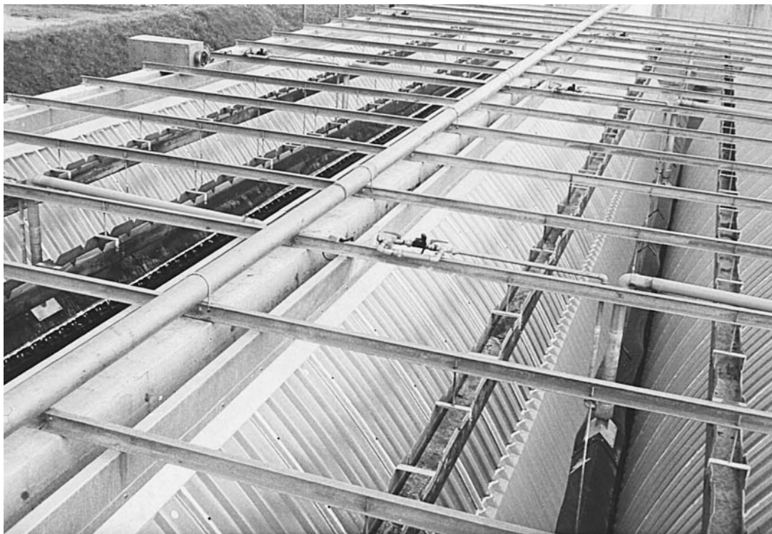
Fig. 10.11. Picture of chemical USBF reactor 2 \times 250 L/s. Coal mine Svatava, Czech Republic.
