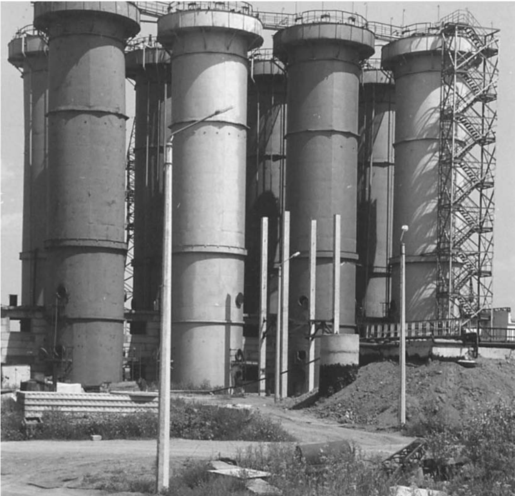
Fig. 9.4. View of actual combined column-type design of wastewater treatment plant manufactured from steel, including the primary settler, column aeration tank-clarifier, tertiary filter with the gravel media, capacity—22, 000 m 3 /day.
