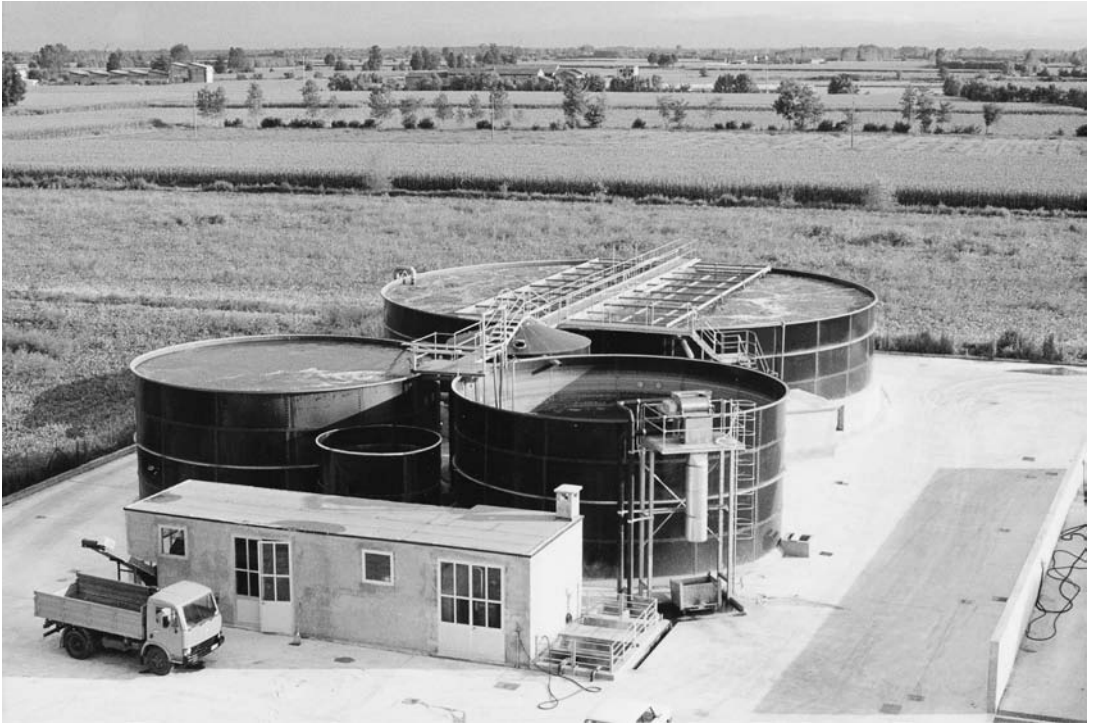
Fig. 10.19. View of a slaughter house WWTP Pro Sus, Italy ( 1000\text{ m}^3/\text{day} ).
