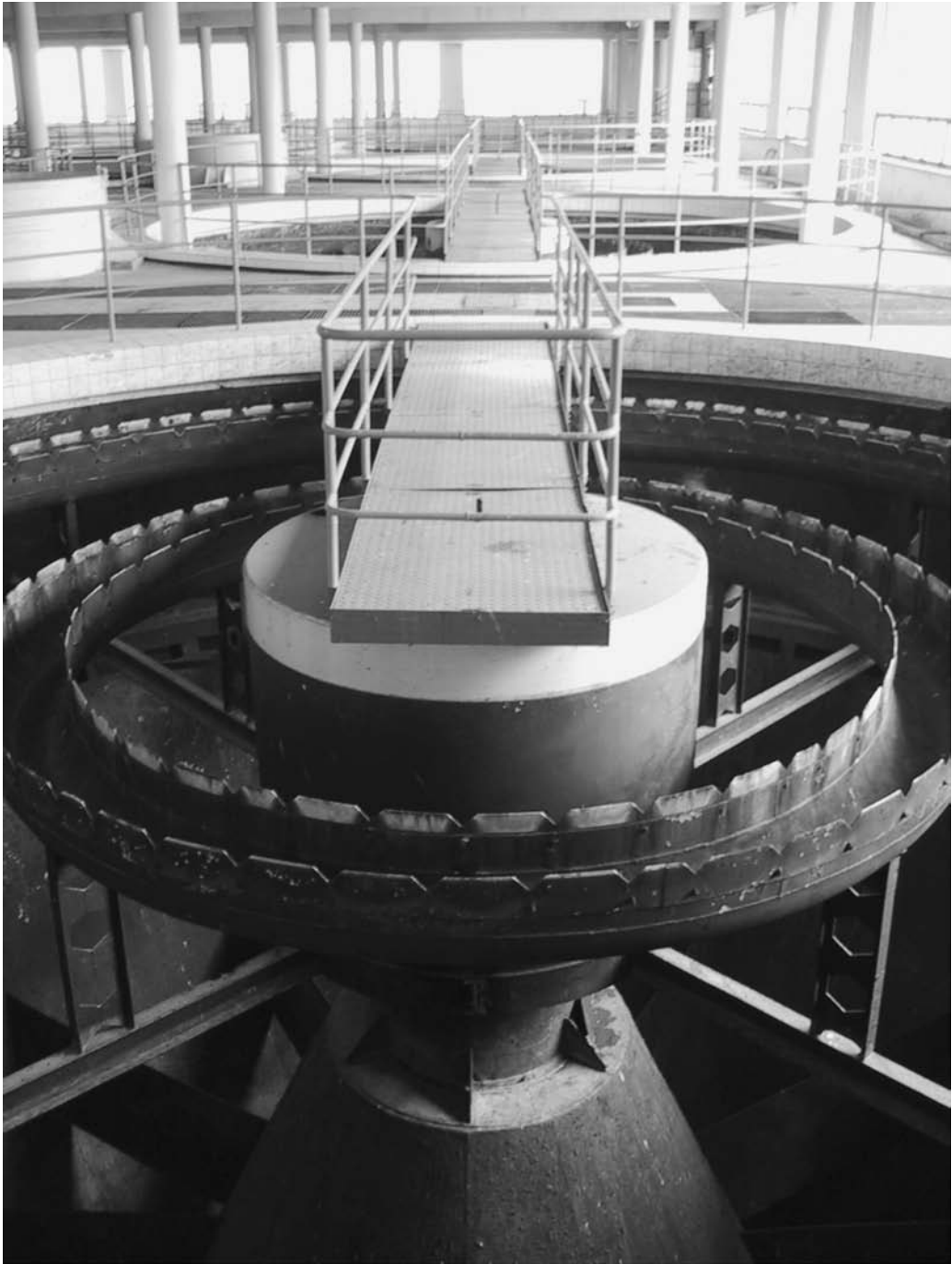
Fig. 10.9. Inside view of Municipal Treatment Plant for potable water with total capacity 1000 L/s ( 8 \times 125 L/s). Brno, Czech Republic (1956).
