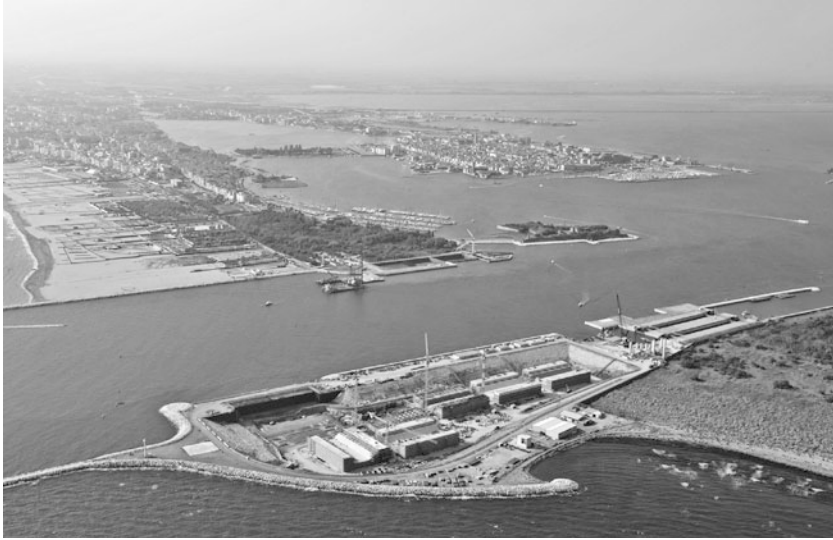
Figure 6.2 The Chioggia, one of the three inlets that connect the Venetian Lagoon and the Adriatic Sea. In the foreground, the temporary gate housing caisson prefabrication site and the double lock for fishing boats and emergency vessels. In the background, Chioggia. Credit: Ministry of Infrastructure and Transport—Magistrato alle Acque (Venice Water Authority), concessionary Consorzio Venezia Nuova image archive.
