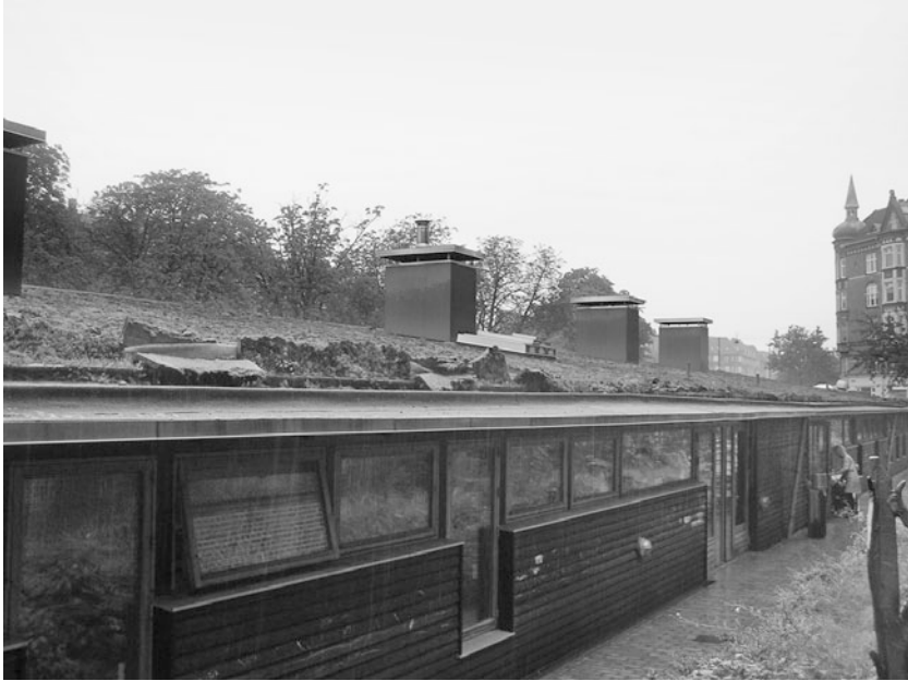
Figure 4.5 A city-run ecological kindergarten, designed and constructed under Copenhagen’s new green building standards. Credit: Bergit Jorgensen.
