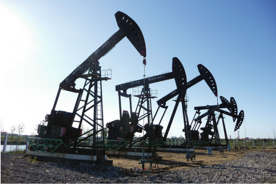
Fig. 15.1 Six of the thousands of pumpjacks of Daqing move in a rhythmical ballet as they lift oil to the surface from the oilfield. At the moment I captured this “ballet step” I decided that if I was ever to write a book about oil then this image would be in it (Photograph by Kjell Aleklett)
