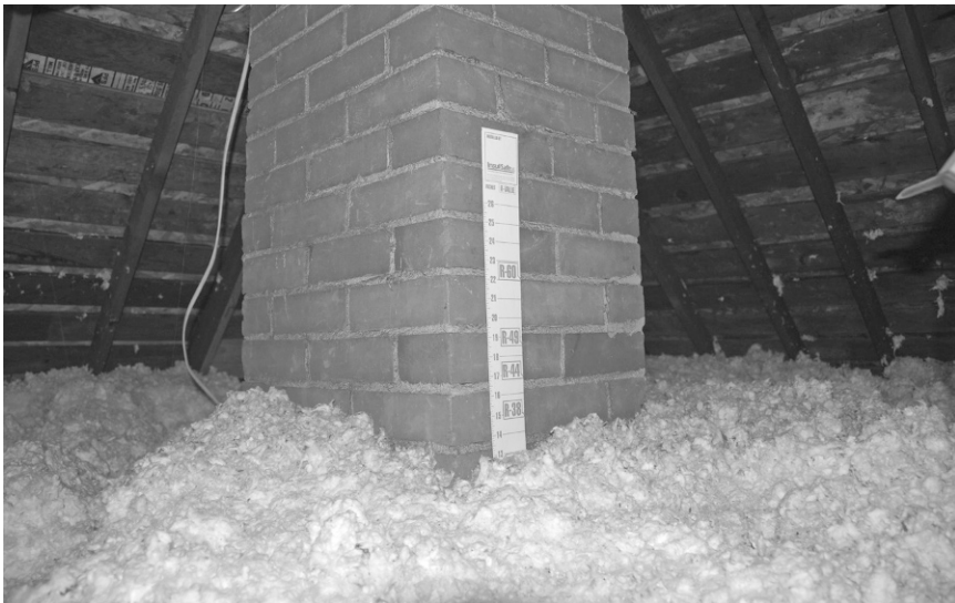
Figure 3.27. For residential buildings, insulating the attic floor is an effective way to reduce heat loss. This loose insulation, originally rated R38, has settled, as indicated on this installation gauge.
