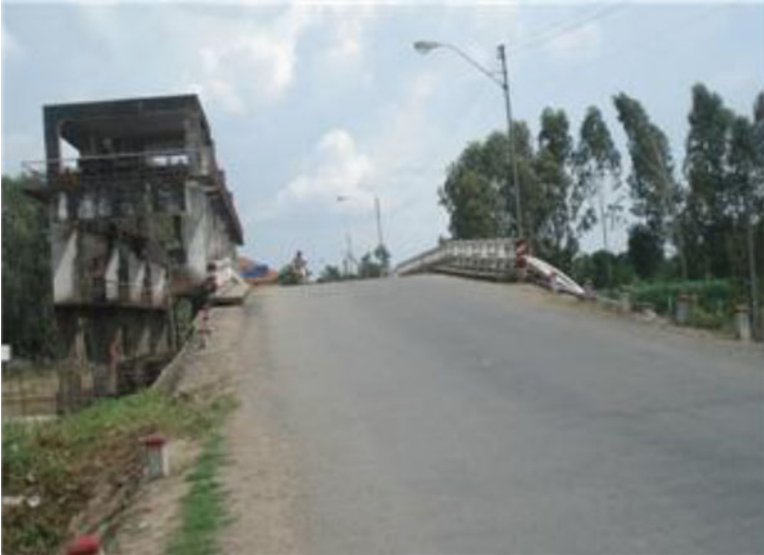
Fig. 10.17 Sluice gate and dyke system under the framework of South Mang Thit sub-project (Source: own picture N.T. Binh 2010)
