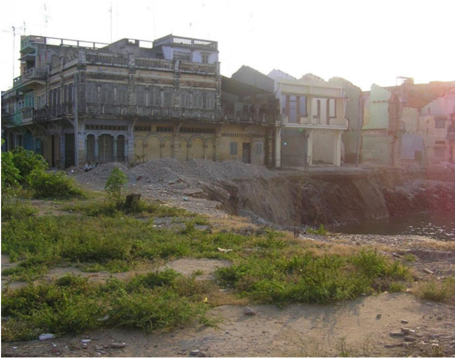
Fig. 3.14 River bank erosion in the Tan Chau District (Hung and Ngoc 2004)
