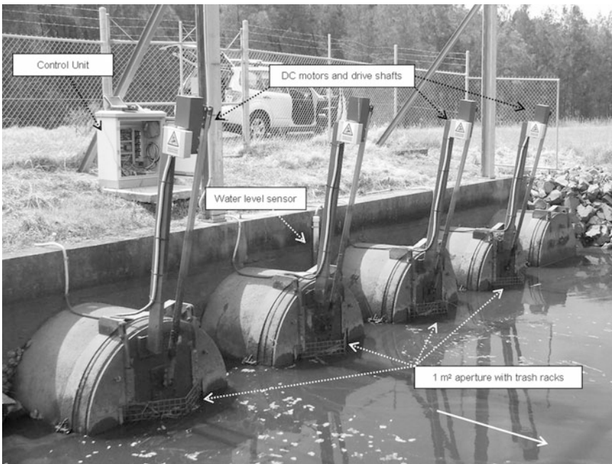
FIGURE 17.5. Example of multiple SmartGate units. Components of the SmartGate are indicated (dashed arrows). The solid white arrow indicates ebb tide flow direction.
