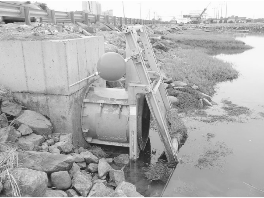
FIGURE 21.1. Self-regulating tide gate (SRT), Route 1A in Revere, Massachusetts, adjacent to the Pines River. Unlike conventional flapper tide gates, which provide drainage flow only through a top-hinged structure, the SRT is a float-actuated water control valve that uses a bottom float to open the gate on incoming tides. A second set of adjustable floats (the round floats in this photo) on the valve allows the gate to close for flood protection. (Photo courtesy of Edward Reiner).
