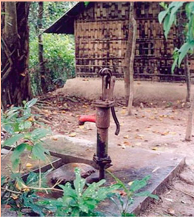
Box Fig. 3.2a.2 Tubewell with red painted spout indicating high arsenic content in the water, Chittagong District, Bangladesh, 2000 (Photo credit: S. Hanchett)
