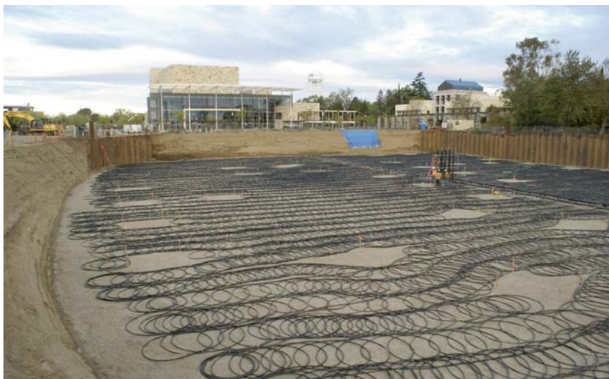
Fig. 7.4 Construction of geothermal ground loop system to provide heating and cooling (Credit: Bovis Land Lease)
