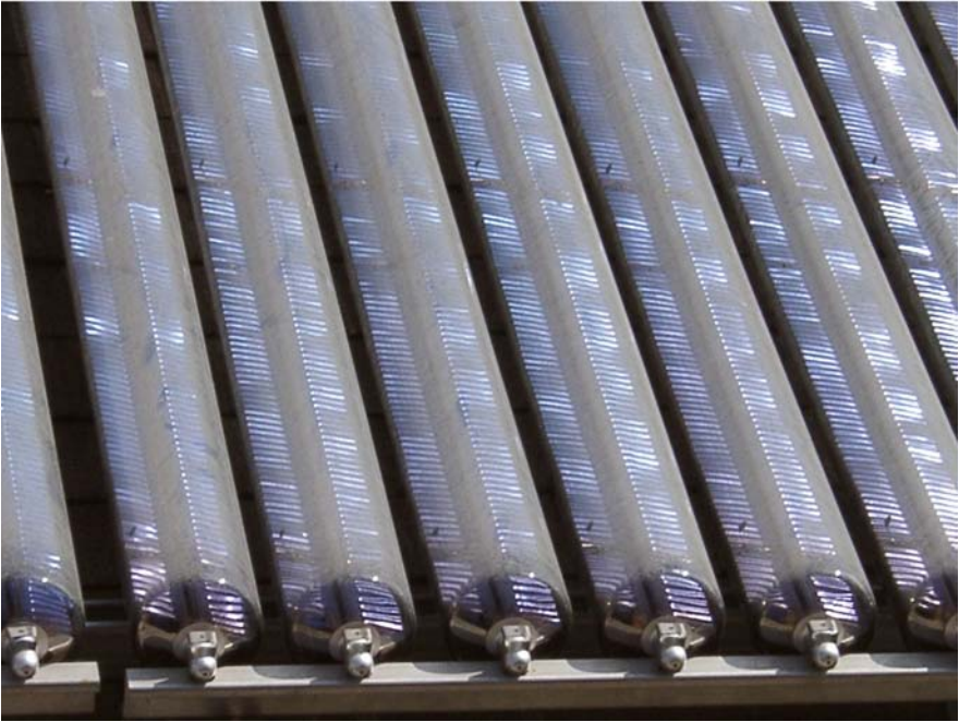
Solar heat pipe technology used for heating/cooling at Audubon Center
