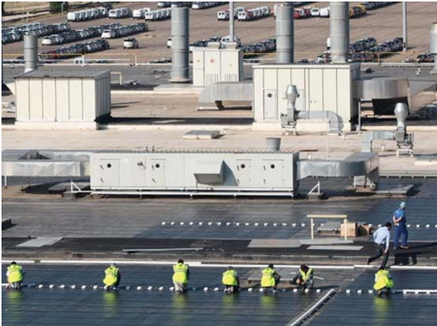
Solar array being installed on a General Motors assembly plant in Zaragoza, Spain
