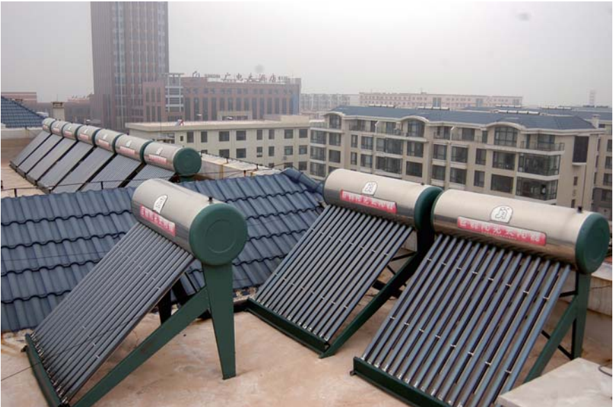
Fig. 14.4 Closeup view of rooftop of solar thermal water heaters in Rizhao, China [5]
