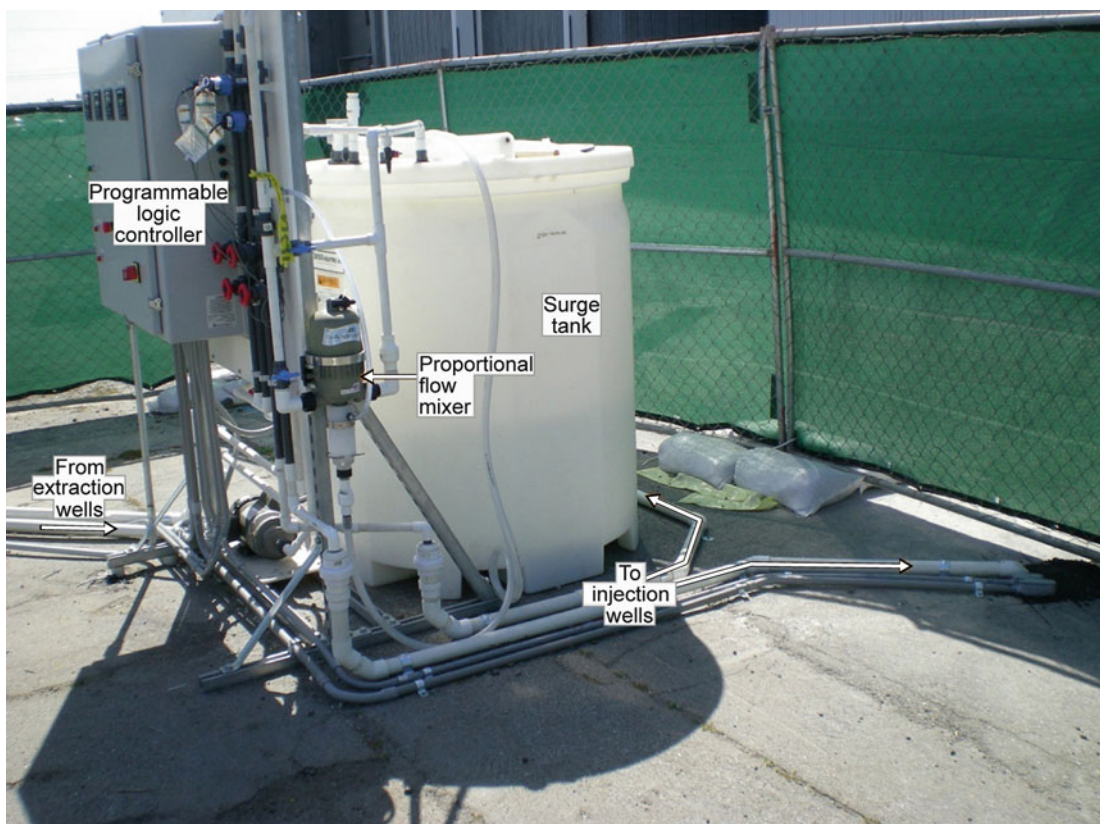
Figure 5.4. Photo of an active recirculation bioremediation system.
