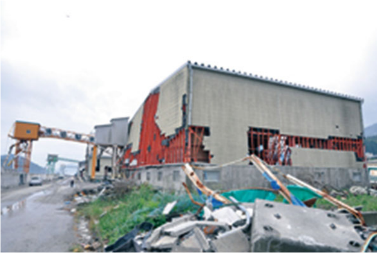
Fig. 3.3 Destroyed ice works facility near a fishery harbor (Source: MAFF)
