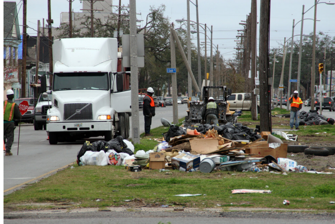
FIGURE 6-2 New Orleans, Louisiana, February 24, 2006—FEMA contractors remove debris created by Hurricane Katrina from the Lower Ninth Ward. Crews continue collecting wreckage throughout the neighborhood as more people return to rebuild New Orleans. Robert Kaufmann/FEMA.
