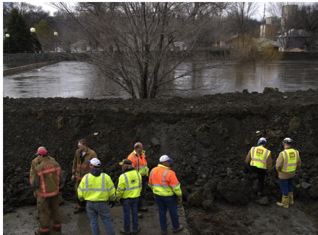
FIGURE 3-4 Valley City, North Dakota, April 13, 2009. Members of the U.S. Army Corps of Engineers inspect the site of a levee where severe seepage threatens the integrity of the levee in downtown Valley City, North Dakota. The Corps is working with city officials and the National Guard to ensure the safety of the levees in the town. Photo by Patsy Lynch/FEMA.
