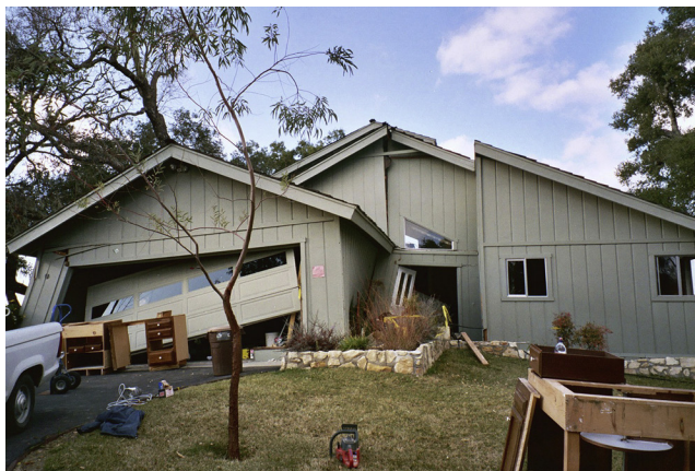
FIGURE 2-3 Atascadero, California, January 25, 2004. This home slid 2 feet off its foundation due to the 6.5 San Simeon earthquake. Photo by Dane Golden/FEMA News Photo.
