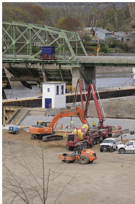
FIGURE 7-2 Glensville, New York, April 18, 2012—Infrastructure on Lock-9 of the Erie Canal system on the Mohawk River is being repaired for flood control systems announced by Governor Andrew Cuomo as part of a state-wide works project. FEMA plays a vital role supporting state, tribal, and local governments as they respond with recovery efforts. Hans Pennink/FEMA.
