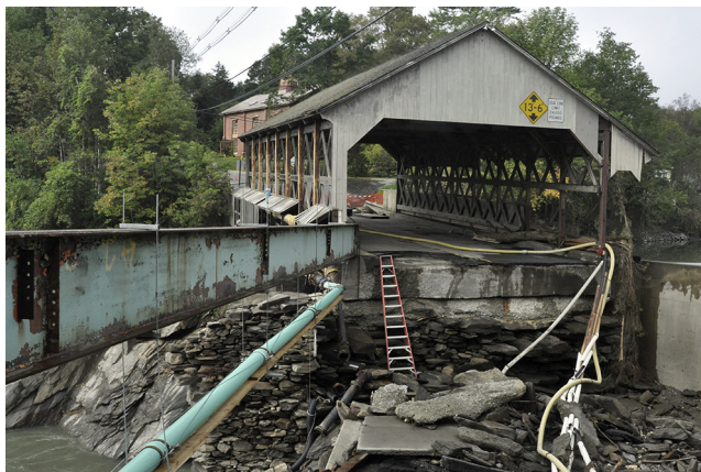
FIGURE 2-2 Quechee, Vt., September 11, 2011—The Quechee bridge is a main thoroughfare and an integral part of the town. Residents cried as they watched their beloved bridge battered by flash flood waters caused by tropical storm Irene. Photo by Wendell A. Davis Jr/FEMA.
