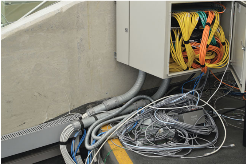
Fig. 12 Loose wires in the Maracanã, 2015
