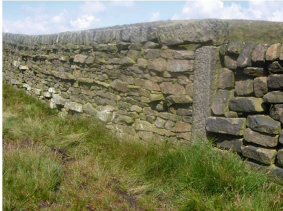
Fig. 23.5 Well-built parliamentary enclosure wall with three lines of throughstones and well-laid capstones, Trawden
