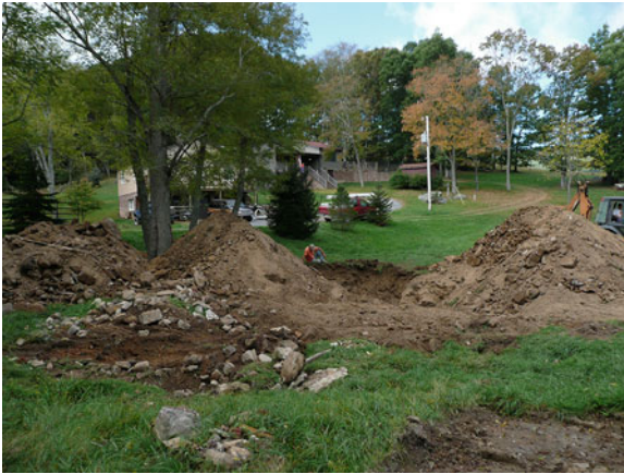
Fig. 13.1 The Landrum’s yard after the first round of excavations. Photo by P. C. Lucas
