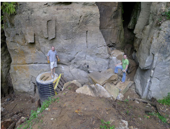
Fig. 11.41 Brad Cooper on the completed double pipe and concrete entrance and Nathan Farrar on the rubble formed by pulling down the fractured pillar (photo by P. C. Lucas)
