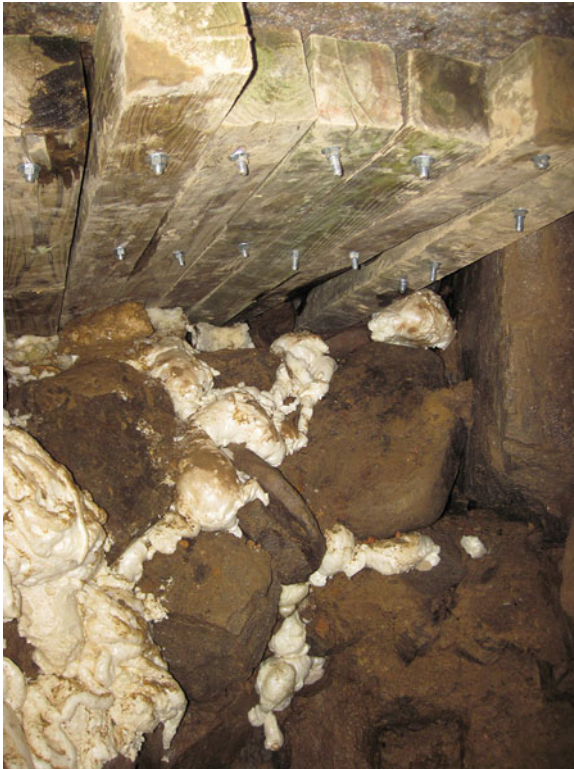
Fig. 13.18 Timber roof supporting loose rocks with foam stabilizing other loose rocks. Photo by Y. M. Droms
