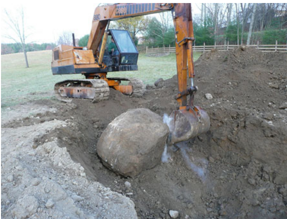
Fig. 13.7 Excavation of big rocks with Paul Cunningham’s track hoe. Photo by P. C. Lucas
