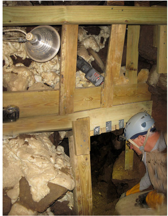
Fig. 13.19 The stabilized Bowling Ball Wall. Photo by N. C. Farrar
