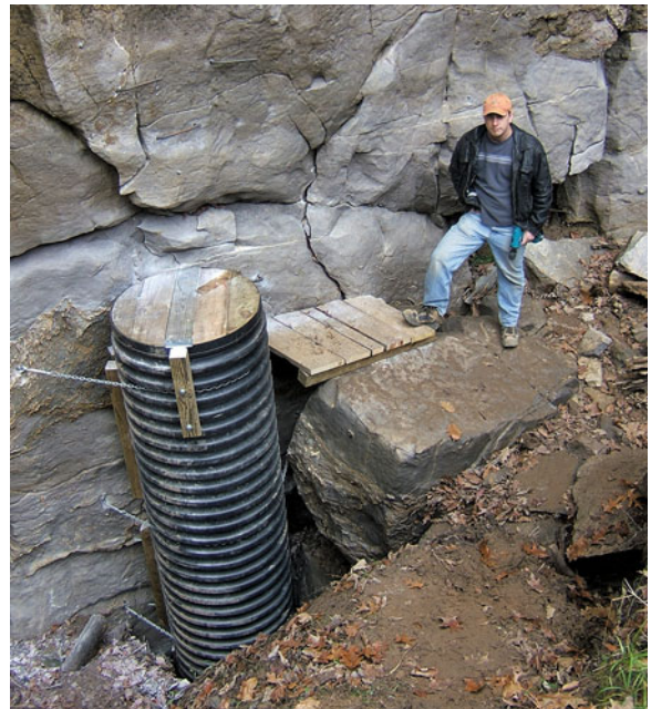
Fig. 11.11 Matt Lucas at the top of the new Subway culvert pipe entrance that is chained to the cliff (photo by P. C. Lucas)
