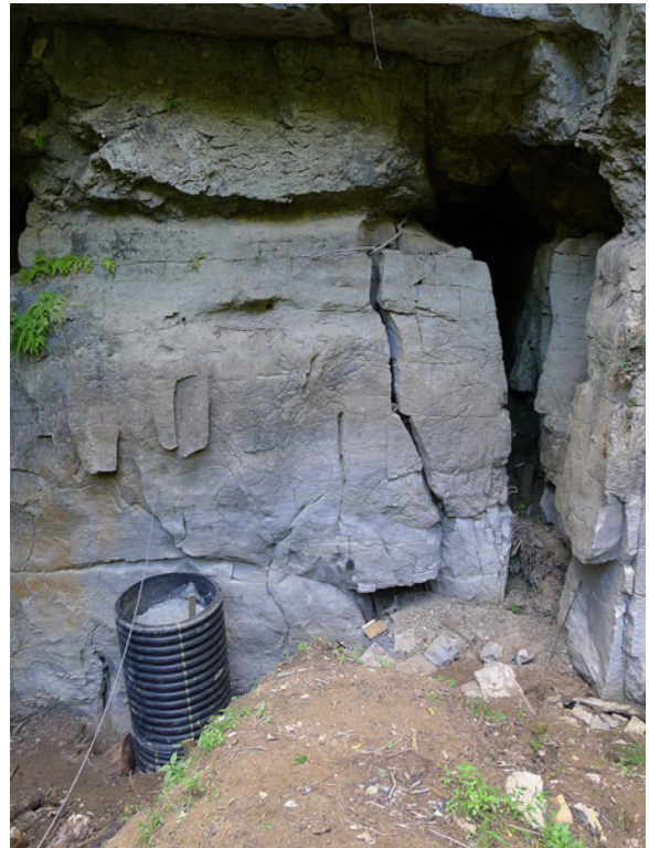
Fig. 11.40 The inner pipe of the entrance and the crack in the limestone pillar (photo by P. C. Lucas)
