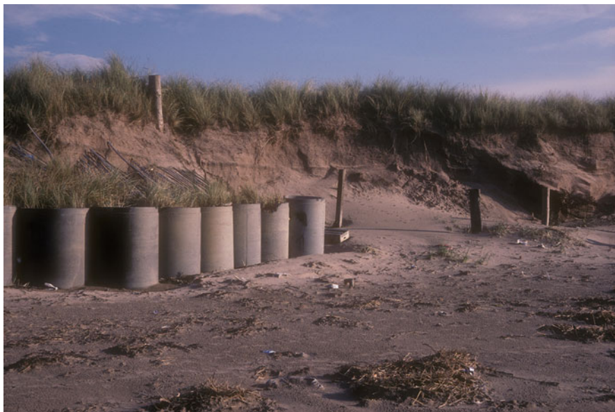
Fig. 10.6 Foreshore along the southwest facing sand dune of the Royal Troon, January 1991. The picture shows erosion outflanking the concrete pipes filled with sand, installed to prevent loss of part of the golf course
