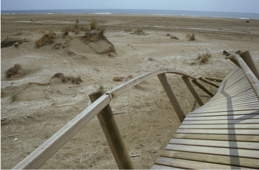
Fig. 6.3 Eroding dune front, Ebro Delta, Spain. The walkway over the sand dune has collapsed as the dune has eroded, September 1996
