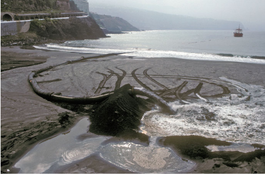
Fig. 9.4 Beach nourishment using volcanic sand to create an amenity beach in Tenerife, 1995. Material is pumped onshore via a pipeline from an offshore vessel
