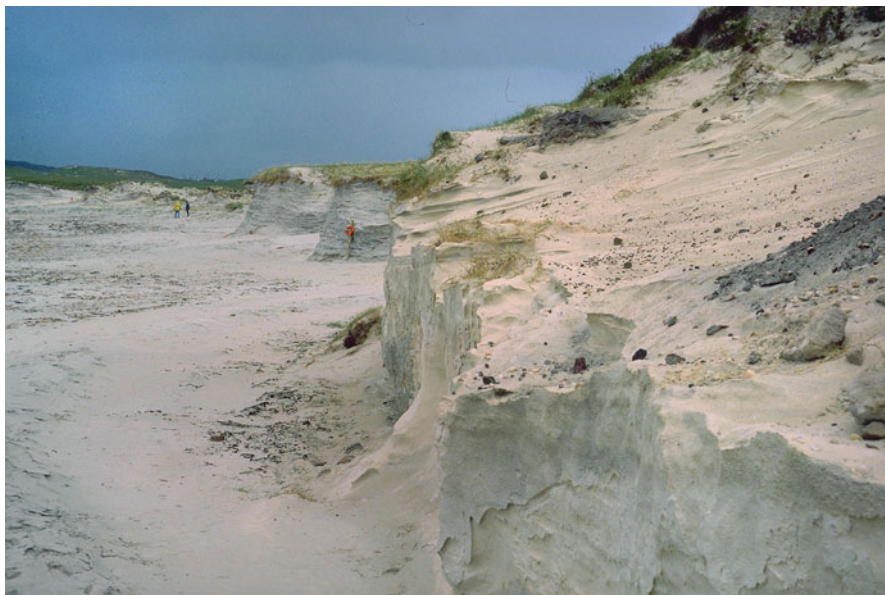
Fig. 11.7 Eroding and under-cutting of the machair surface on the west coast of Ireland. In this location relative sea level rise is implicated. Heavy grazing, recreational activity, sand extraction and exposure combine to cause loss of surface vegetation and erosion of the sand. The sand cliff in the foreground is approximately 3 m high, July 1991
