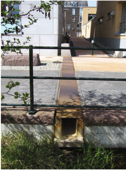
Figure 2.16. Storm-water outlet to canal in Boo1. (Photograph by Bengt Persson.)
