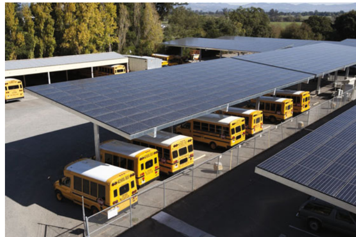
Figure 7.8. View of photovoltaics over a parking structure. ( Photograph by Sunpower Inc. )
