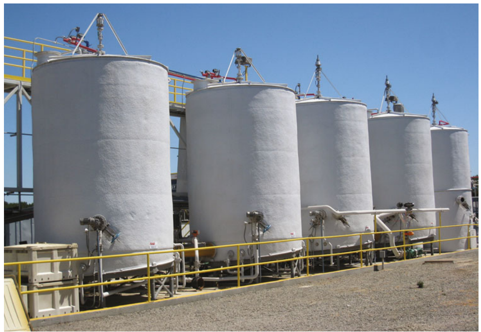
Figure 7.27. View of biodigester in West Village. (Photograph by the University of California, Davis.)
