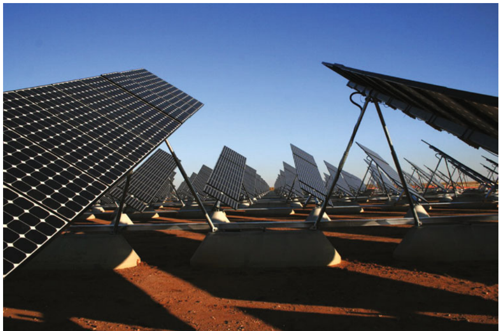
Figure 7.3. View of solar farm. (Photograph by Sunpower Inc.)
