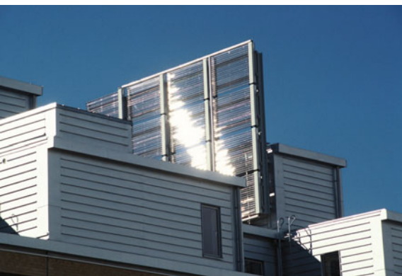
Figure 2.20. View of evacuated tube collectors in Boo1. (Photograph by Jan-Erik Andersson.)
