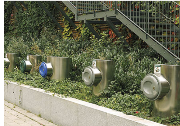
Figure 3.25. View of vacuum waste system stations in Hammarby Sjöstad. (Photograph by Lennart Johansson.)
