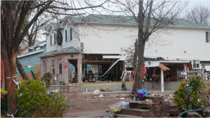
Fig. 2.7 A home partially destroyed by Super Storm Sandy, Staten Island, New York (Photograph by author, 2012)
