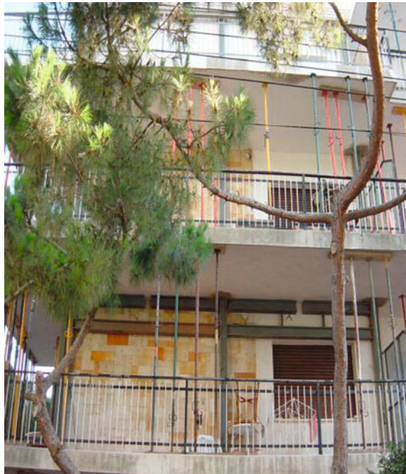
Fig. 2.5 Shoring of balconies in vacation homes in Playa d’Aro, Spain (Photograph by author, 2003)
