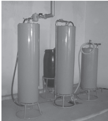
Figure 5. Water Purification System Developed for Rural Areas of the Aral Sea Region (Height of the Largest Column Is 2,400 mm).
