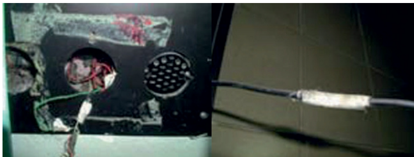
Figure 1. Typical wiring infrastructure at a hospital in Kosova.
