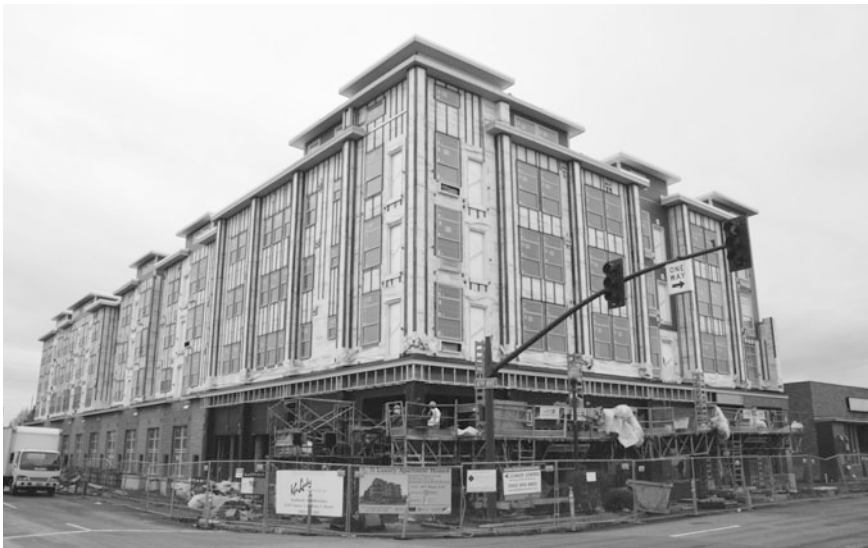
Figure 4.2b. Nearing completion in 2014, the main bank building (far right) was preserved and converted into retail space, and seventy-one residential units with ground-floor retail were constructed on drive-through lanes and most of the parking. Parking access is behind the buildings. (Credit: Tokola Properties)
