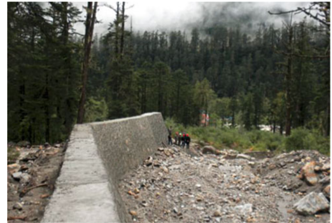
Fig. 4 Design sketch map and completed anti-impact wall at Key Section 1 of Huangbengliu debris flow
