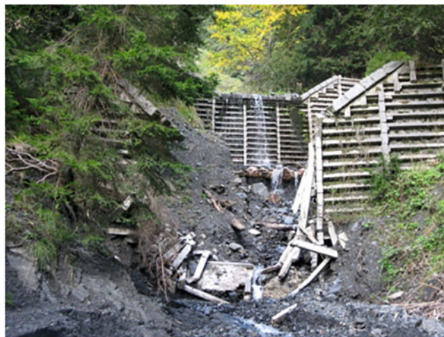
Fig. 4 Example of a collapsed check dam
