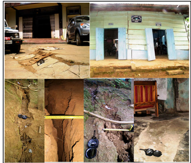
Fig. 4 Photograph of some of the transverse cracks in New Colony
