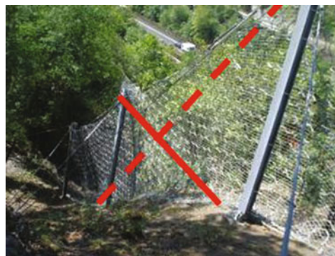
Fig. 5 Example of a difference in post elevations which may modifies the barrier behavior because it induces anomalous stress conditions: low stress in one direction of the panel ( continuous line ) and high stress in the other one ( dash line ). Location: Autostrada A22—km 62 + 640 and km 63 + 150, Bolzano (Ita)
