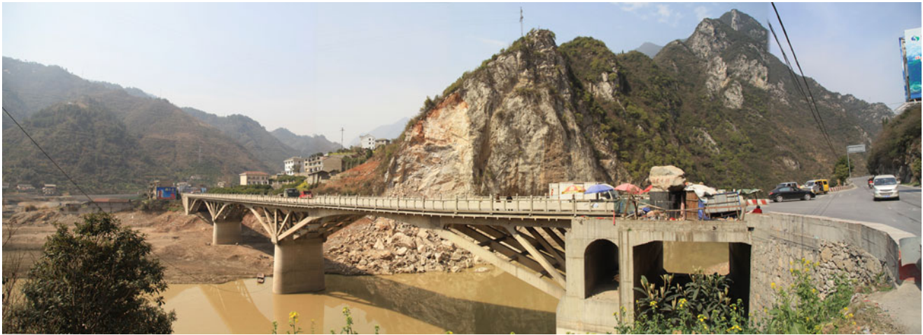
Fig. 2 Overview of the Zhaojun Bridge Rockfall
