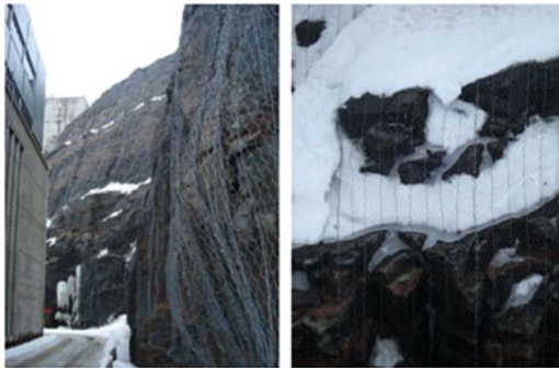
Fig. 8 Detail of the simple drapery system installation. Left : limited space between the slope and the hydro-power generation station; Right : detail of the snow accumulation on the mesh
