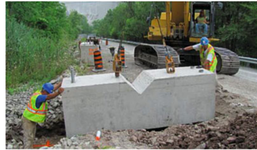
Fig. 1 Installation of large steel-reinforced-concrete plinth for a post foundation. The barrier’s energy level is 2,000 kJ. Location: Niagara Falls (ON, Canada)
