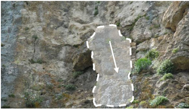
Fig. 9 Rock slide failure detected along the slope face
