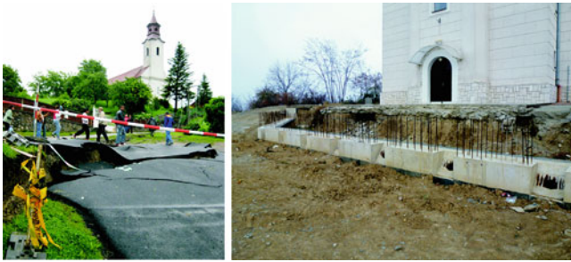
Fig. 5 View from the bottom to the St. Mathew church in the central part of Nižná Myšľa Village and to local road damaged by the landslide ( left ) as well as to bolted pile wall under construction (Photo: L'. Petro, 4th June 2010/24th November 2011)
