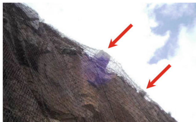
Fig. 6 Example of a heavy drapery (HEA cable panel, weight > 2.0 kg/m 2 ): the mesh is able to keep in place the blocks along the slope (red arrows)
