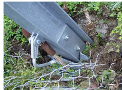
Fig. 9 Settlement of a footplate after the impact. The displacement was approx. 0.2 m vertically, and 0.1 m horizontally to downslope, km 425 highway A3 (2011)
