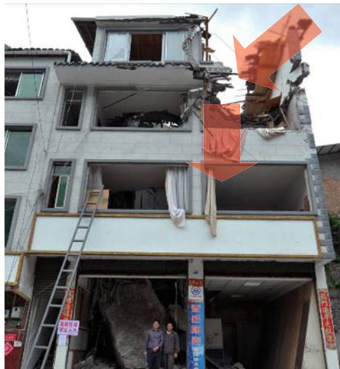
Fig. 6 Houses destroyed by rock falls in Baoxing
