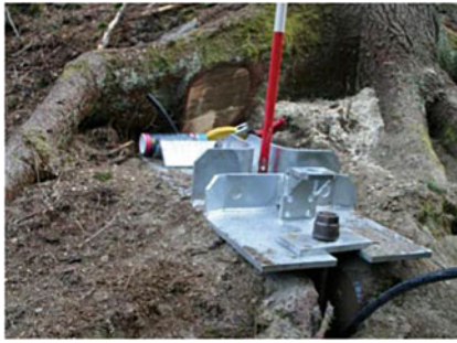
Fig. 2 Light foundation: the steel footplate is directly lying on soil and tree roots without any plinth. The barrier has energy level of 3,000 kJ. Location: Kirchstrasse, See (Austria)
