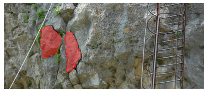
Fig. 8 Small size rockfall in the lower portion of the pillar
