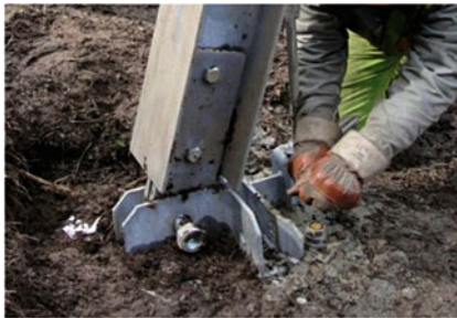
Fig. 3 Installation of the post on the footplate directly lying on soil. The barrier has energy level 3,000 kJ. Location: Kirchstrasse, See (Austria)
