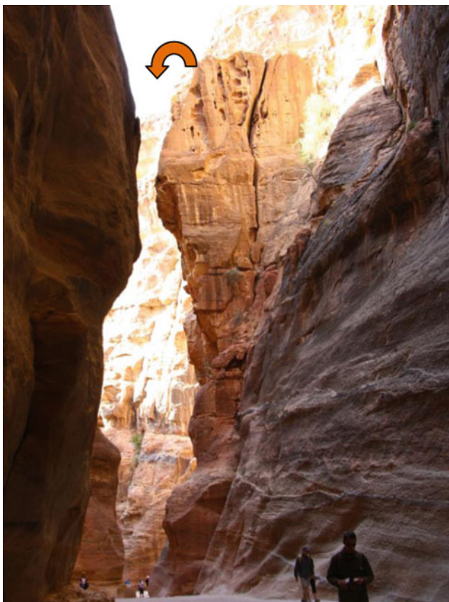
Fig. 6 Potential toppling failure mode of a large block
