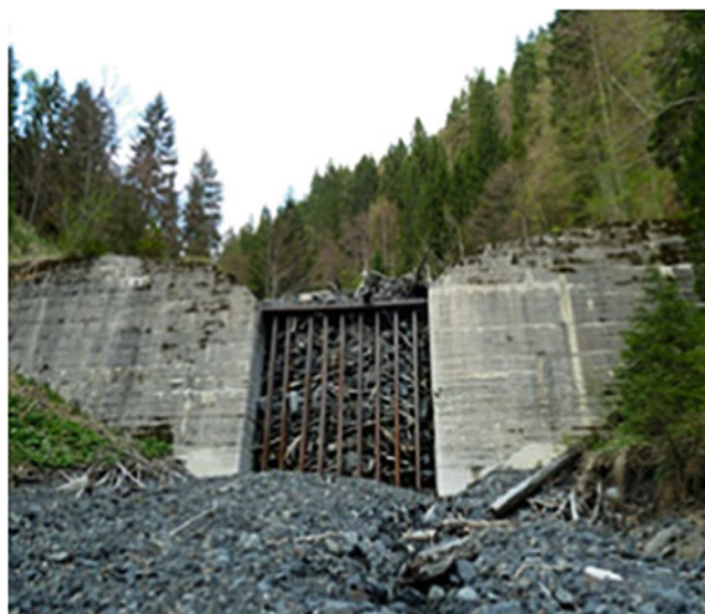
Fig. 5 Example of a filled concrete check dam in the Suhelj Torrent with a filtering function
