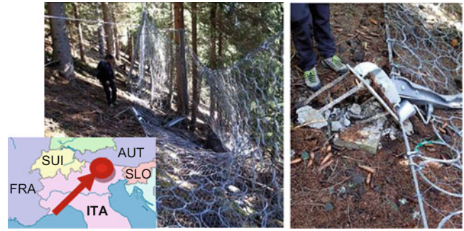
Fig. 11 Effect of the impact against the post of a 2,000 kJ barrier. Location: Colle Santa Lucia (Belluno, Italy—2013)
