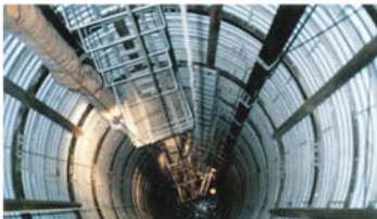
Water catchment well
