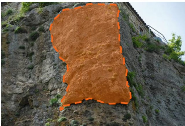
Fig. 10 Unstable rock masses in the upper portion of the pillar
