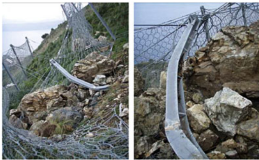
Fig. 7 Effects of the large impact on the primary barrier, at km 425 of the highway A3 (2011—Italy). The post is 6 m long
