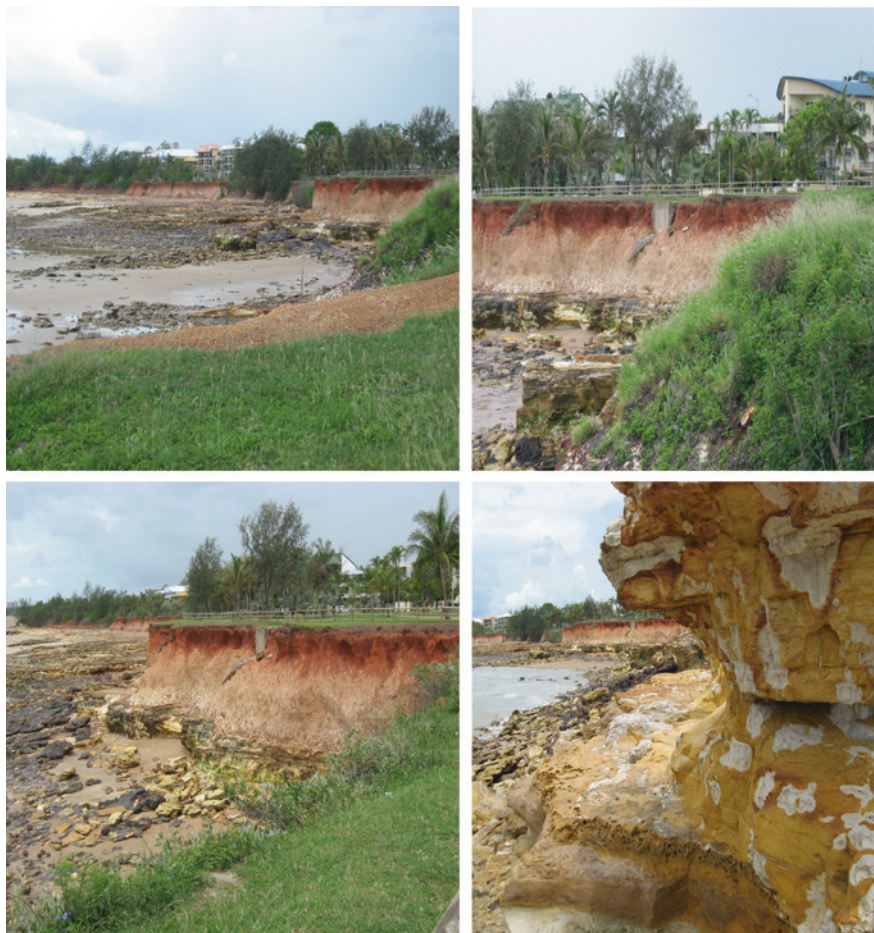
Fig. 5.15 Erosion from surface runoff and large stormwater outlet-Nightcliff ( top ), complete cliff erosion ( middle ) and serious coffee rock cliff erosion close to apartments ( middle and bottom ), yellow sandstone-dolomitic layer ( bottom ) (Jones et al. 2008)
