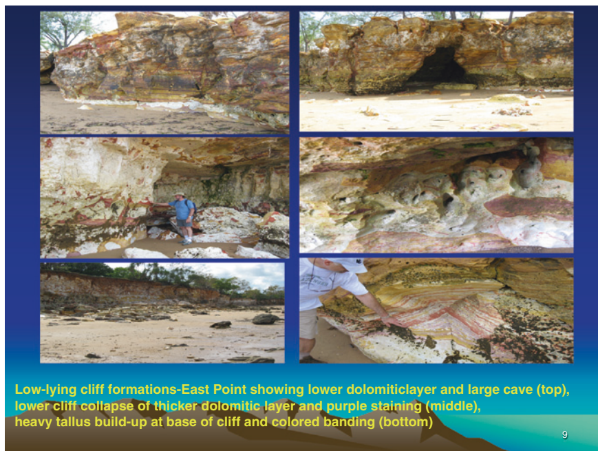
Fig. 5.14 Cave formation at East Point aligned in westerly orientation to ocean waves ( top ), erosion due to freshwater flows from cliff top ( middle ), erosion along deep cracks and joints; and collapsed section of cliff ( bottom ) (Jones et al. 2008)
