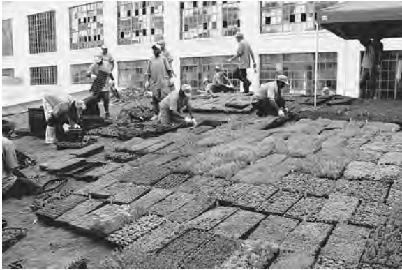
Figure 3.14 A greenroof ready to plant, showing porous-aggregate lightweight planting mix. (Project: Emory Knoll Nursery. Photo: Ed Snodgrass.)
