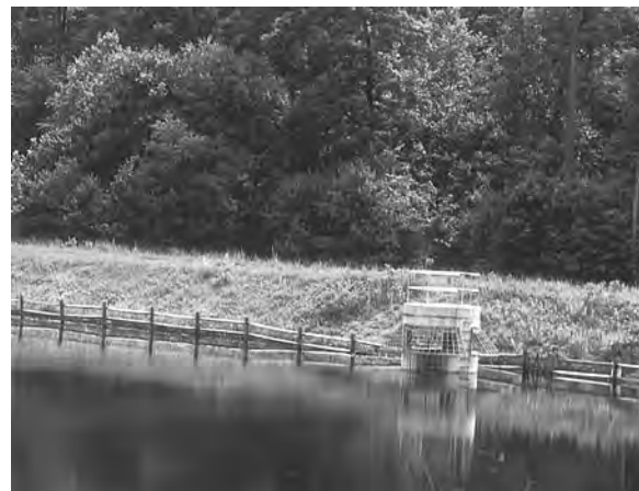
Figure 4.9 The T-shaped opening in this wetland structure sets the water level. Small rises in level flow out through the “trunk” of the T; if major flooding raises the level higher, the top of the T permits faster drainage. (Project and Photo: Rick Scaffidi, EQR.)
