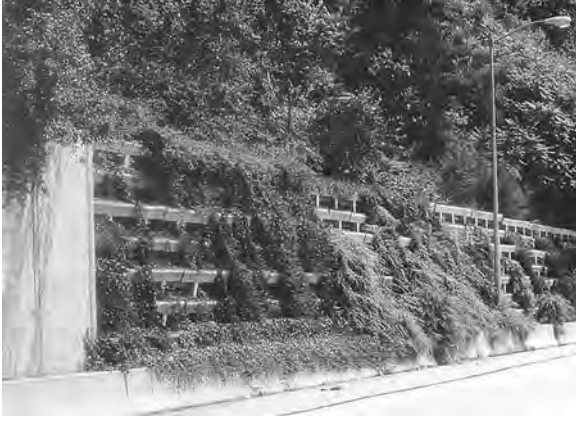
Figure 3.9 The Evergreen “trough” greenwall serves both as retaining wall and as noise wall on Philadelphia’s Blue Route (I-476). (Project and Photo: Synterra Ltd.)
