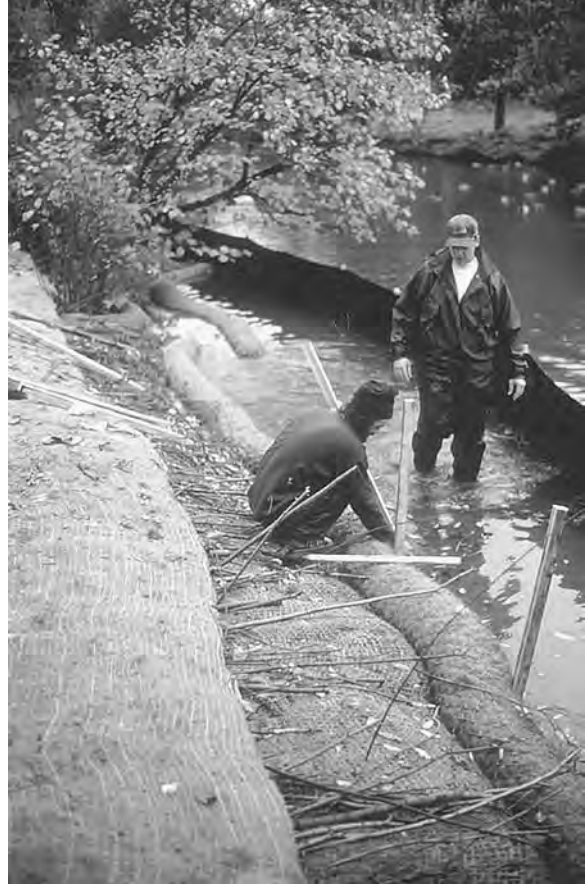
Figure 4.14 Students installing “burritos” and brush-layer to stabilize the stream bank. ( Project and Photo: Professor Stan Jones.)
