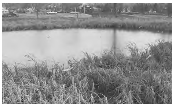
Figure 4.10a,b,c This constructed wetland was (a) excavated to careful depths required by wetland plants, then (b) lined. Planted with marsh-tolerant sedges (c), the completed wetland treats graywater organically for re-use, reducing this Michigan convent’s water use by half. (See p. 202 for project description.) (Project and Photo: Veridian Landscape Studio.)
