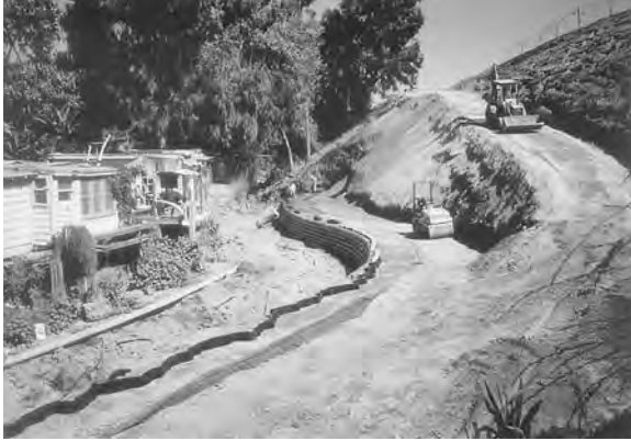
Figure 3.12a,b Greenwalls can reduce the “footprint” or horizontal extent of a high bank by steepening it. This approach protects Crystal Cove State Park (California) from increased upstream runoff—shown during and after construction. (Project: California State Parks, Steve Musillami. Photo: Alan Tang.)
