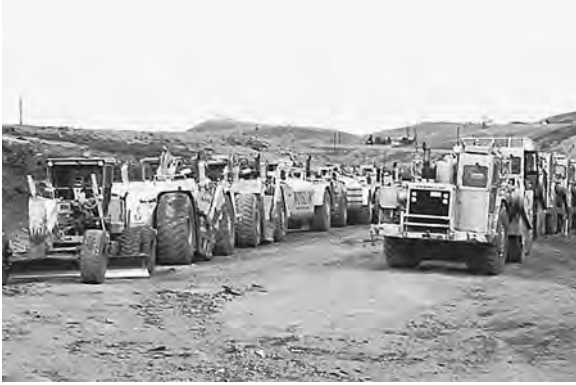
Figure I.12 Staging areas (this one is for a fairly small road project) can permanently damage an expanse larger than the site of actual work. (Photo: Kim Sorvig.)
