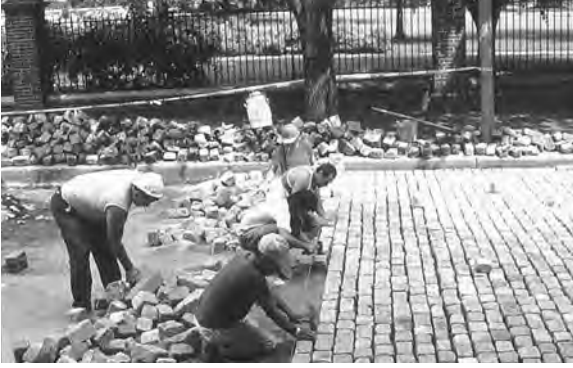
Figure 5.II Traditional granite setts being laid on sand in Philadelphia’s historic district. Joints are somewhat permeable if not mortared. (Photo: Kim Sorvig.)
