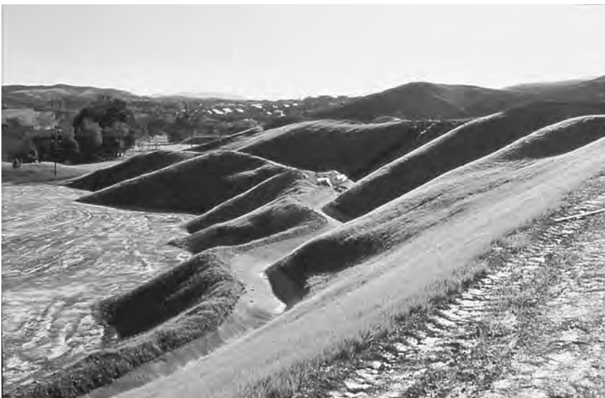
Figure 2.9 Landform grading creates forms that resist erosion by being in equilibrium and that increase habitat diversity and aesthetic appeal. Lifetime costs of creating and maintaining these forms is less than conventional grading. (Project and Photo: H. J. Schor.)
