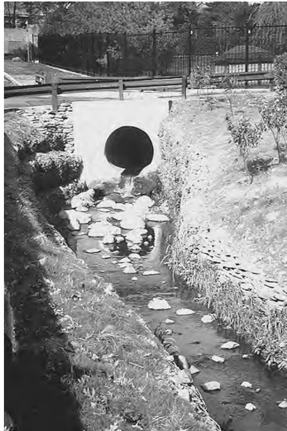
Figure 4.19 Maguire Avenue after installation of gabions, boulders to deflect culvert outflow, and plantings. (Project: New York City Department of Environmental Protection. Photo: Dean Cavallaro.)
