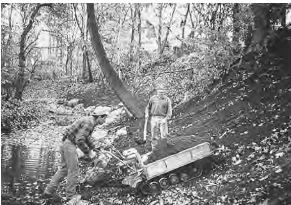
Figure 7.5 Motorized wheelbarrows, like this Honda PowerWagon, can do heavy work with decreased site impact, as in Sweet Brook's restoration. (Project: NY DEP. Photo: Dean Cavallaro.)
