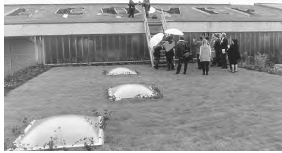
Figure 3.19 The ecoroof atop Ecover's headquarters helps meet the company's goal of a green factory producing green products. (Project: Ecover. Photo: Peter Malaise.)
