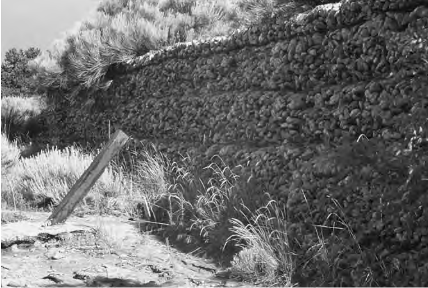
Figure 3.8 Gabions cause fewer problems than impervious walls because they allow water to seep through. Over time or by design, gabions can support vegetation. (Photo: Kim Sorvig.)
