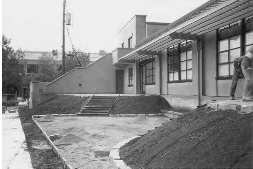
Figure 6.7 The Monnens Addis renovation in progress. (Project: Miller Co. Photo: Jeffrey Miller.)
