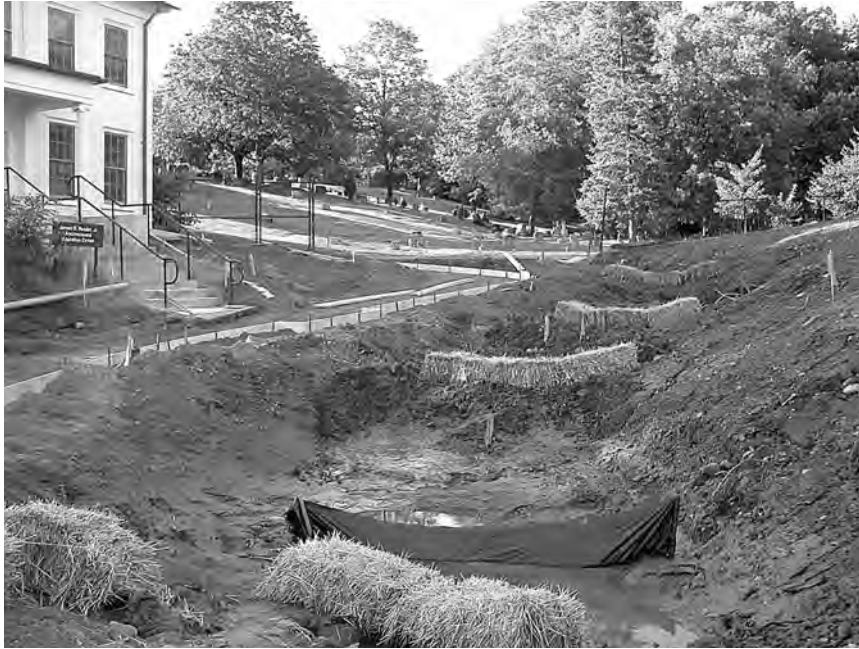
Figure 4.7a,b,c The Nichols Arboretum (Ann Arbor MI) creates beauty from stormwater management structures. The sequence shows construction and planting of stepped pools to control runoff. ( Project: The Nichols Arboretum. Photo: Robert E. Grese. )
