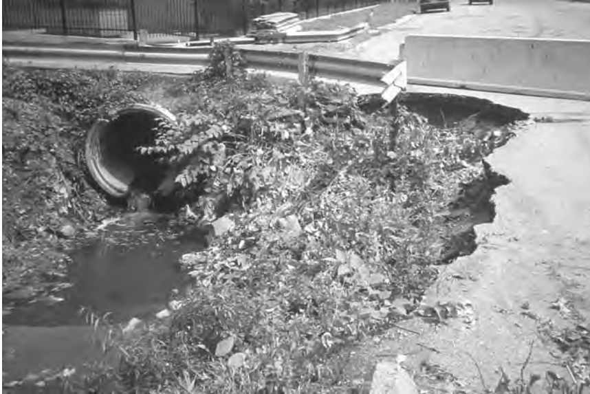
Figure 4.18 Erosion undercut pavement at Maguire Avenue and prevented plants from reestablishing. (Project: New York City Department of Environmental Protection. Photo: Dean Cavallaro.)
