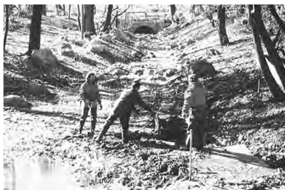
Figure 4.16 Tons of accumulated sediment were removed from Sweet Brook and used to fertilize the restored banks. (Project: New York City Department of Environmental Protection. Photo: Dean Cavallaro.)
