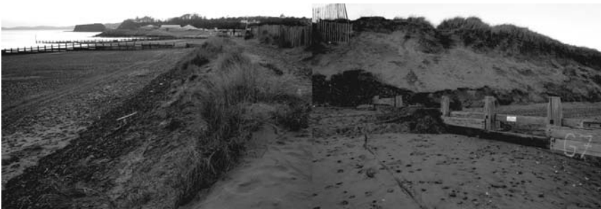
Figure 11.2 (Left) View from Dawlish Warren towards Dawlish showing timber groynes and concrete seawall; (Right) Erosion of sand dunes exposing a rock gabion underlayer at Dawlish Warren
