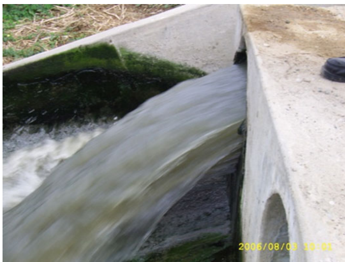
Fig. 8.5 Effluent from the Coloma pumping station
