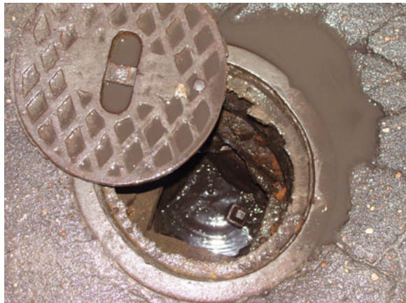
Fig. 15.12 Flooded and filed with sand Riga type hydrant (2 m in deep) due to raised groundwater level
