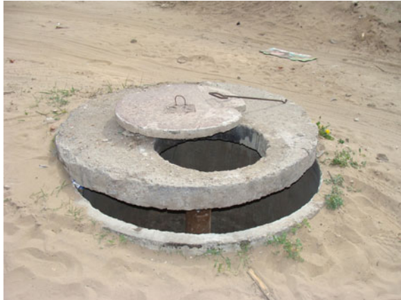
Fig. 15.13 By third person damaged manhole of hydrant in Riga case study
