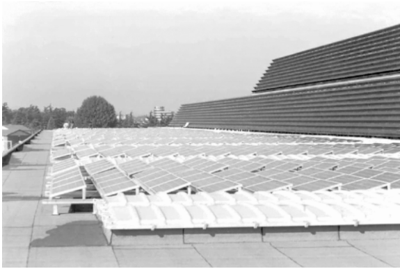
Figure 3. Bologna Airport 80KWp.
