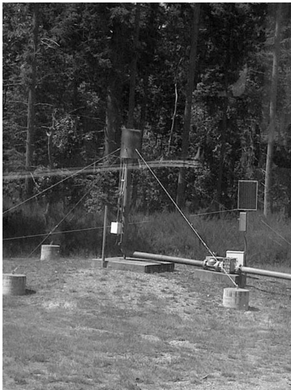
Fig. 13.4 Flare system for landfill gas burning at Joint Base Lewis-McChord
