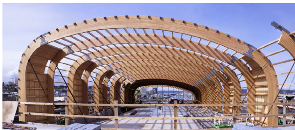
Fig. 8.3 Glulam beams (manufactured by APA Member American Laminators) create the arched curve profile of the roof (designed and erected by Western Wood Structures) of the Lemay Car Museum under construction in Tacoma, Washington, USA. Photograph courtesy APA, Tacoma, USA.
