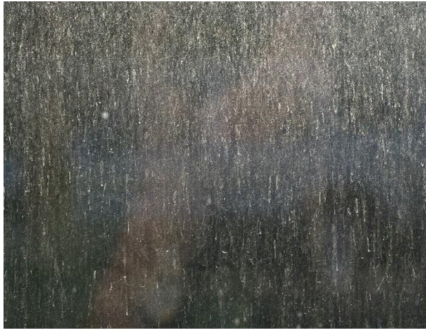
Fig. 5.5 A glass window which has lost optical properties due to the buildup of dirt.
