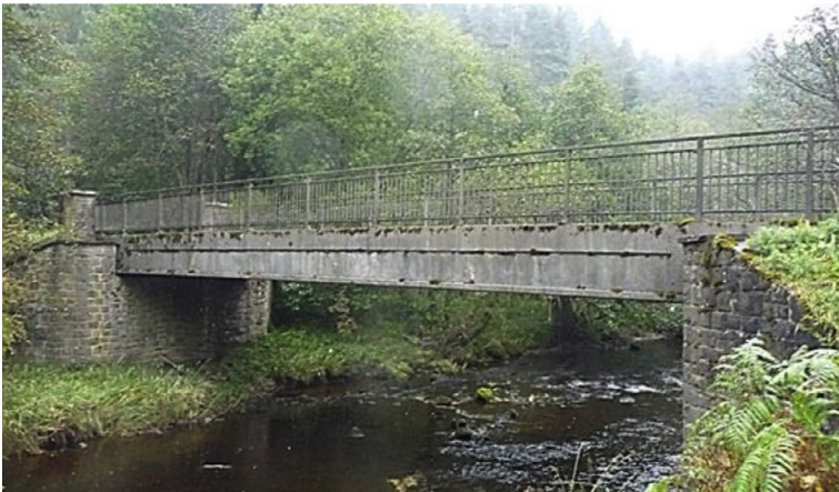
Fig. 10.2 Inverted Tee-beam prestressed lightweight [Lyttag] concrete bridge constructed in 1971, fresh density 1890 \text{ kg/m}^3 , UK Forestry Commission, Redesdale Forest, Northumberland. Philip L. Owens, image 2012.
