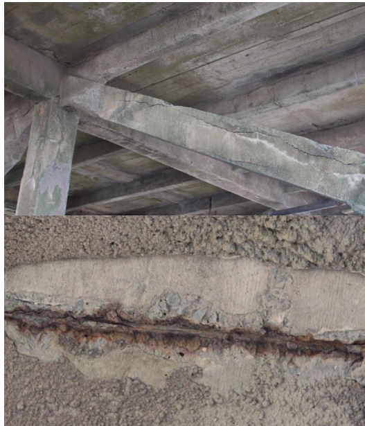
Fig. 16.5 Cracking due to loading and reinforcement corrosion.
