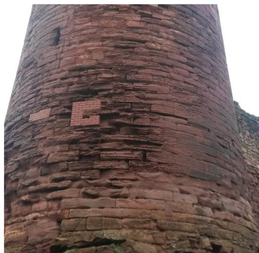
Fig. 12.4 Bothwell Castle (Scotland, UK). Thirteenth-century round tower (south), extensive decay. Temporary stabilisation work evident.
