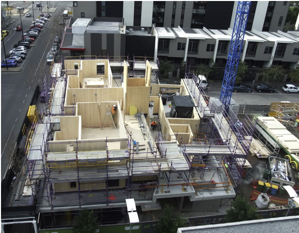
Fig. 8.12 Forté Building under construction. All walls, floors/ceilings are constructed from CLT. Note also the small number of workers on site and minimal crange required.
