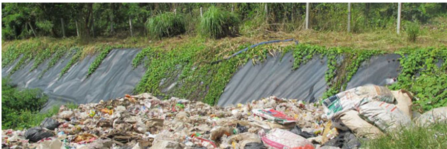
Fig. 4.91 Black rubber silk is laid at the bottom of a landfill. Source Photo by study team
