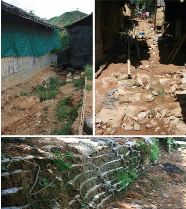
Fig. 4.51 Soil erosion caused by directly pouring wastewater. Source Photo taken by study team
