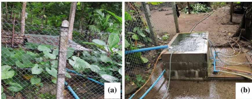
Fig. 4.68 Subterranean course in the shelter area, zone C: subterranean course in the shelter area; and water quality from water supply system. Source Photo taken by study team
