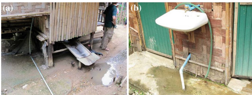
Fig. 4.61 Drainage system from the household: drainage gutter from kitchen and drainage from female toilet. Source Photo taken by study team
