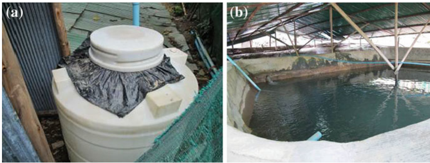
Fig. 4.58 A water quality treatment system, with reservoir for water treatment before distributing to refugee in each spot, and chlorine tank. Source Photo taken by study team
