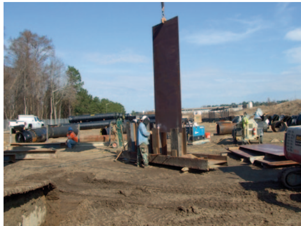
Fig. 3.3 Flat-panel sheet pile vane ready for installation at the Greenville Utilities Commission water supply intake on Tar River, North Carolina, 2012. Only the topmost 1.5–2.0 ft will be above the current bed level. (Courtesy of the Greenville Utilities Commission)
