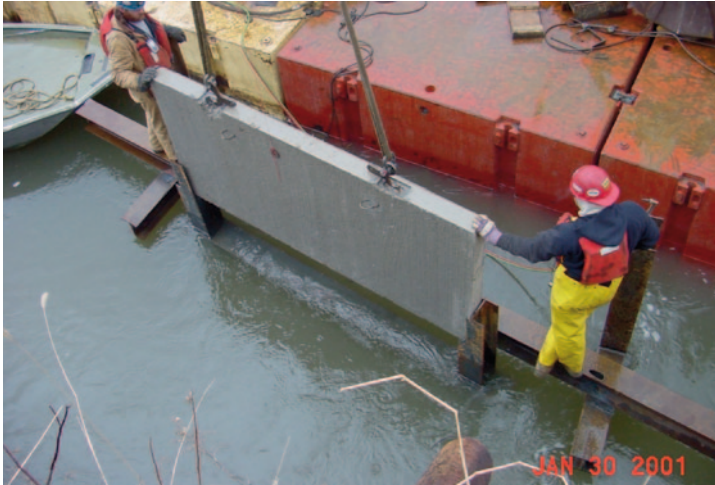
Fig. 3.2 Precast concrete vane panels being placed between H-pile supports. Placement guides extend temporarily above H-columns. (Source: Odgaard [1], with permission from ASCE)
