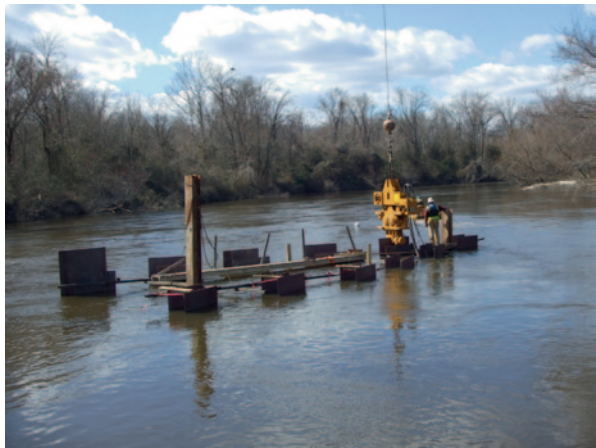
Fig. 3.22 Vanes being installed around intake screens in Tar River, N.C. (Courtesy of the Greenville Utilities Commission)
