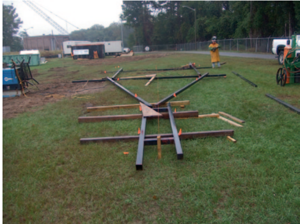
Fig. 3.21 Template used for guiding vane installation at intake screens in Tar River, N.C. (Courtesy of the Greenville Utilities Commission)
