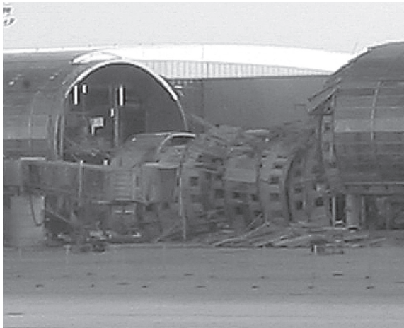
FIGURE 3.3 Partial collapse of Charles de Gaulle Airport Terminal 2E. (From https://upload.wikimedia.org/wikipedia/commons/1/1b/Terminal_2E_CDG_collapse.png . Free licence.)
