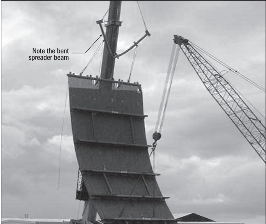
Fig. 9-3. A third-party expert should review lifting or rigging calculations to avoid life-safety issues, not to mention damaged equipment. (Courtesy of Construction Business Associates LLC)
