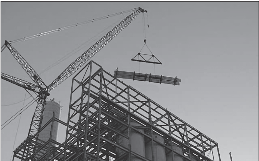
Fig. 7–1. A safely planned lift—there are no personnel below the load. (Courtesy of Construction Business Associates, LLC)
