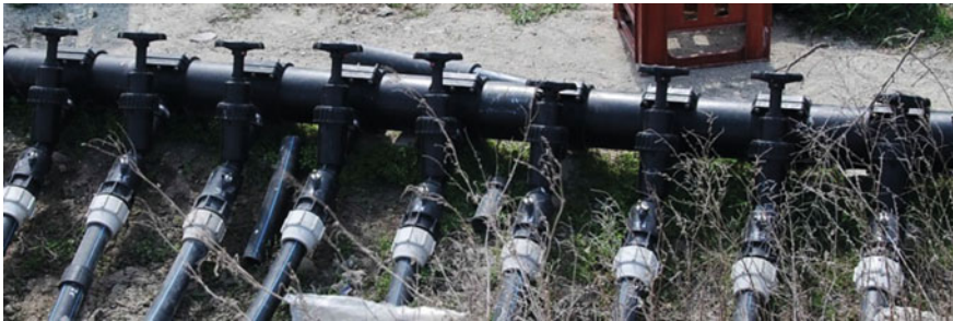
Fig. 3 Collecting point of a gas well pipe network on a landfill. Source own photo
