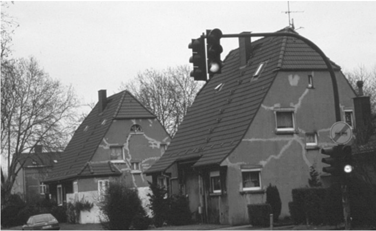
Fig. 6.7 Building damage caused by subsidence of a coal mining area in Gelsenkirchen, Germany
