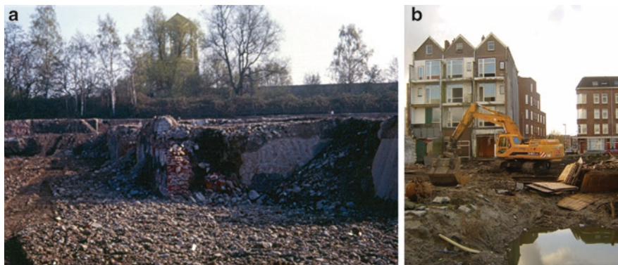
Fig. 5.7 (a) Foundation-soil-mixture of an urban brownfield in Rotterdam, The Netherlands. (b) Demolition residues of an urban brownfield in Rotterdam, The Netherlands
