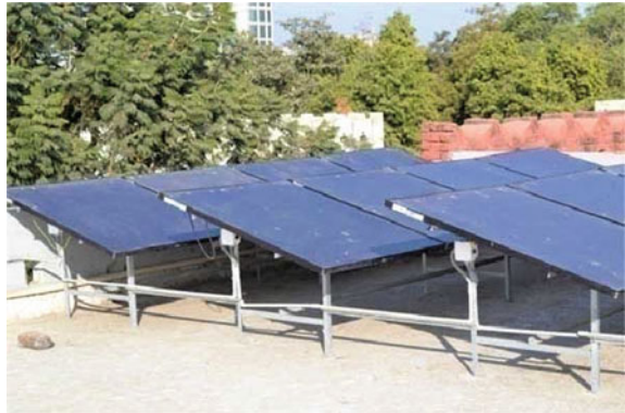
Fig. 4 Solar PV module at the rooftop of one of GV buildings
