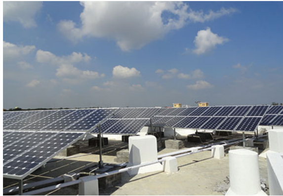
Fig. 1 Solar PV system in the Silver Jubilee Campus. Source Author
