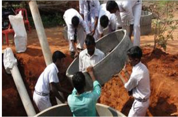
Fig. 7 Student volunteers participating in the building the 7 m 3 Anaerobic Digester, and fencing by felled tree logs available within the campus
