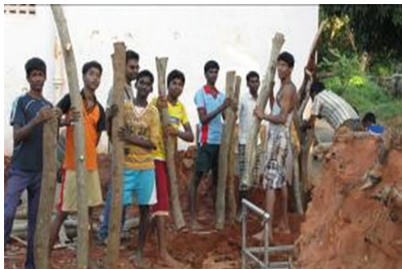
Fig. 6 Student volunteers participating in the building the 7 m 3 Anaerobic Digester, and fencing by felled tree logs available within the campus
