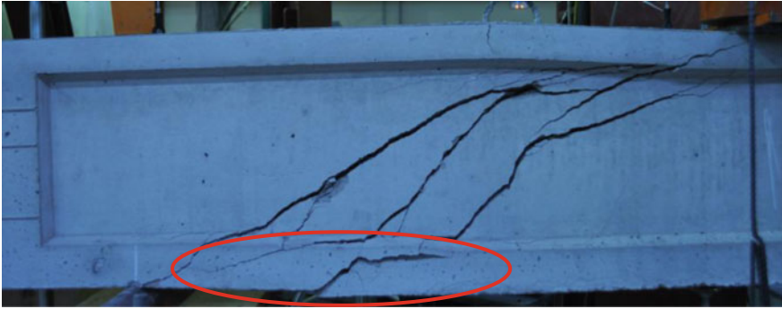
Fig. 6.14 Small cover of beam M-0
