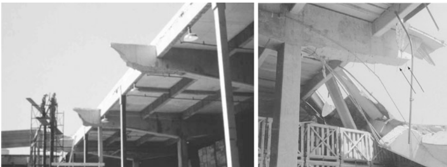
Fig. 1.1 Shear failure of air force warehouse beams ([2, 3] respectively)
