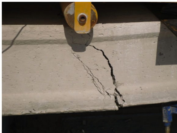
Fig. 7.7 Shear-flexure failure (SF)
