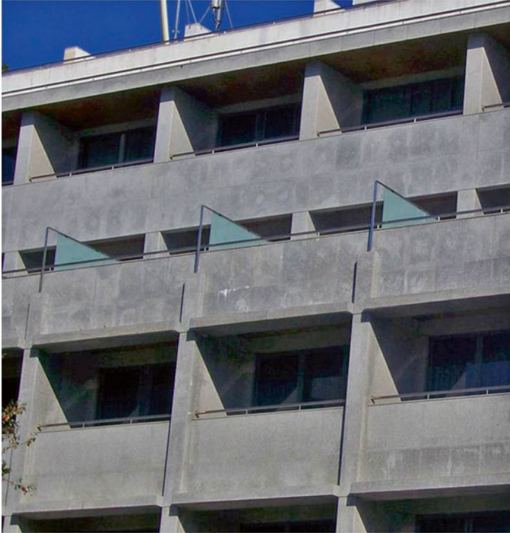
Fig. 1.8 Moisture stains in granite slabs of a façade
