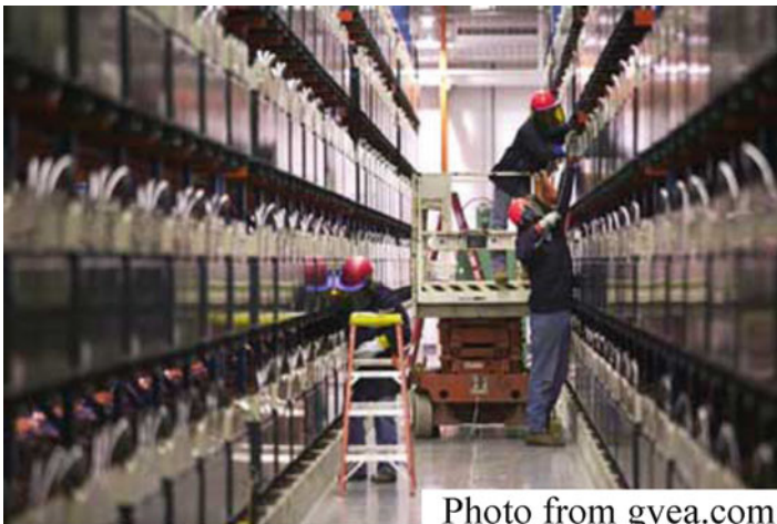
Fig. 2.3 A 27 MW NiCd battery EES system for power grid by Golden Valley Electric Association EES system, Fairbanks, AK
