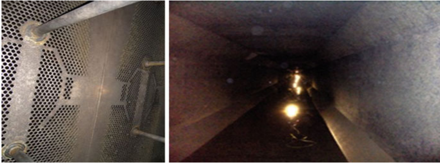
Fig. 8.3 Maasvlakte power station, Unit EFM 1 – return waterbox and intake channel after implementation of Pulse-Chlorination
