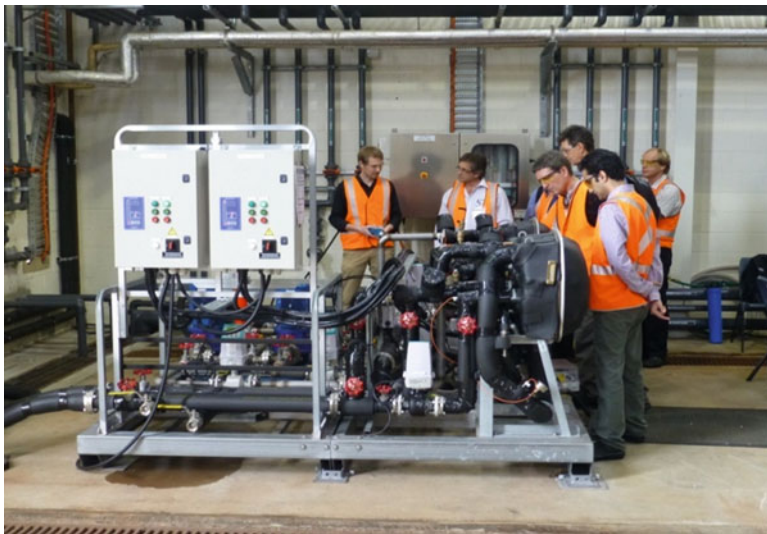
Fig. 12.5 Boosted multi effect distillation pilot plant
