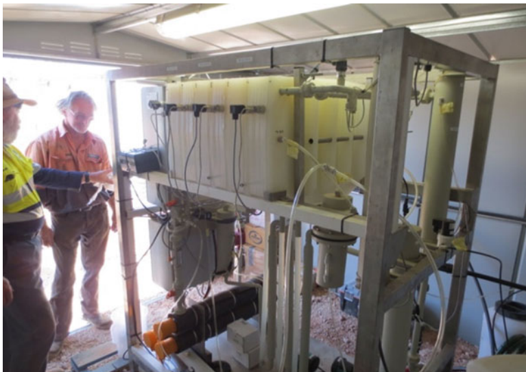
Fig. 12.3 The memSYS VMED unit on site at Tjuntjuntjara
