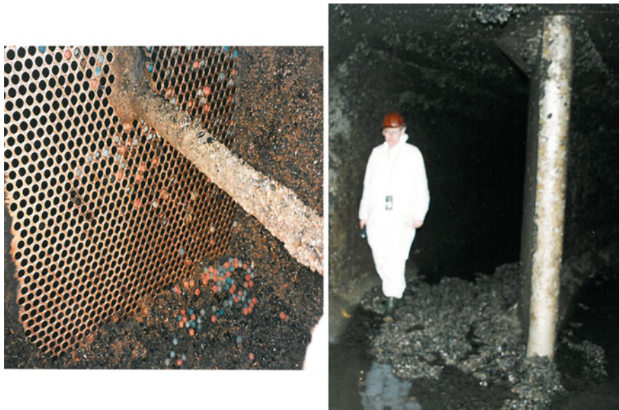
Fig. 8.1 Macrofouling settlements in condenser A (1996) and breach at the intake of the Maasvlakte Power Station, Unit EFM 1. Cooling water intake was last manually cleaned at September 1994. Walls and floor intake channel were covered with mussels in a layer of a maximum 30 cm (Polman et al. 2010)
