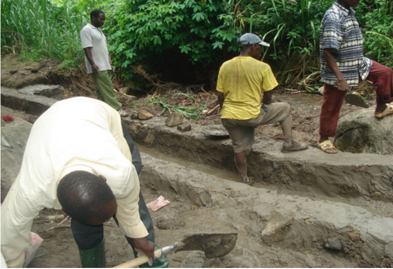
Fig. 9.6 Irrigation canal work in the study area is mainly attended by men
