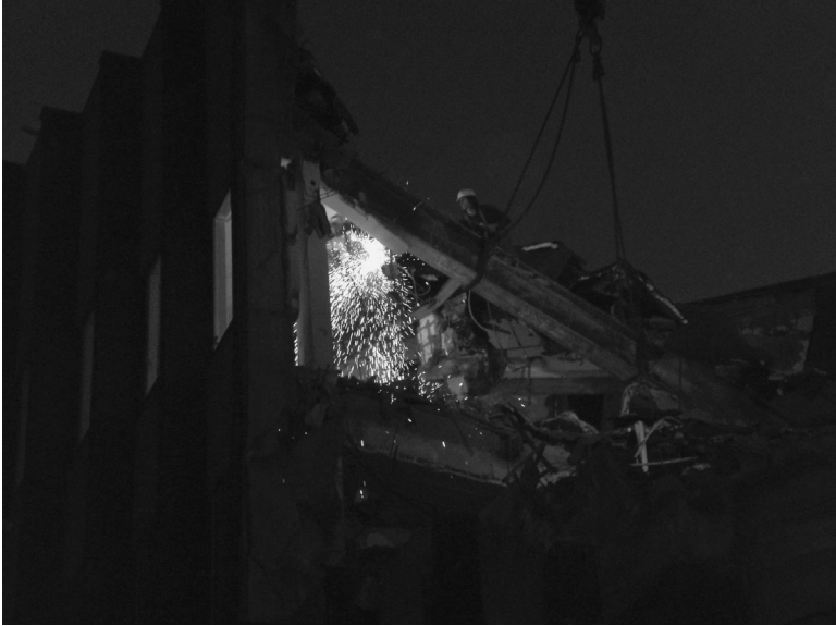
8.12 The beam was flame-cut manually with two bearing cuts and then safely removed by crane.
