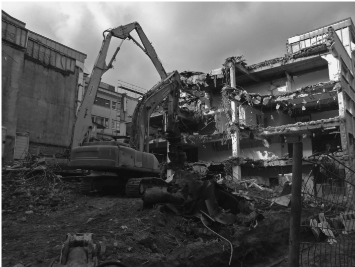
8.9 Typical demolition from top to down: After demolition of all non-bearing structures, the bearing columns are left. In the next step, the columns will be demolished beginning with the top level. After that, the demolition starts again with the next field.
