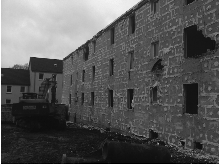
8.14 New materials need the invention of new tools. Deconstruction of insulation plates by an excavator with a newly invented sharp peeler tool.
