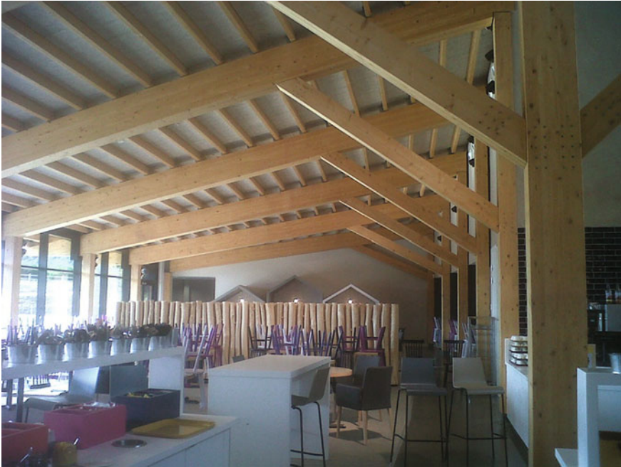
Fig. 7 Some modern buildings may contain large dimension timber structural elements, such as this glulam
