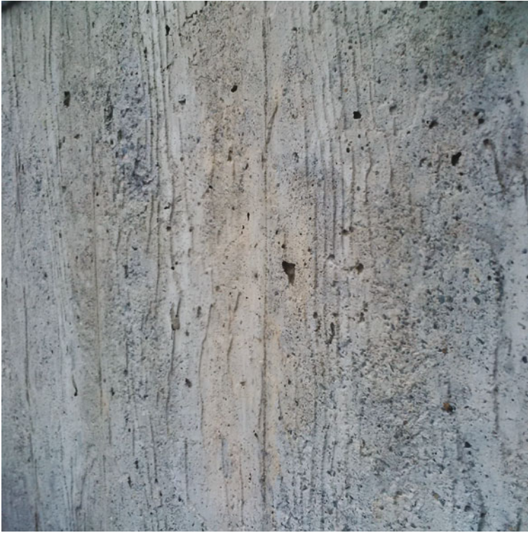
Fig. 6 Wooden false work was used to cast concrete in this 1960s building
