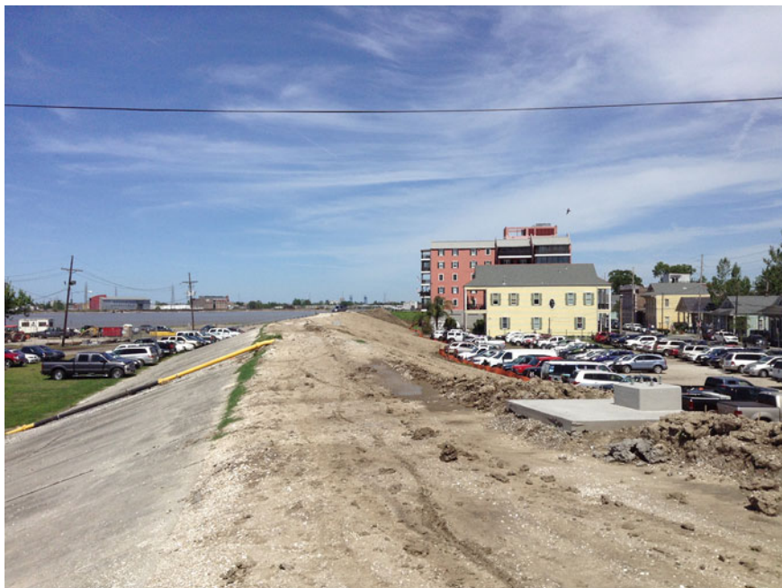
Fig. 1.3 Mississippi river levee at Algiers, Louisiana, directly opposite New Orleans Photo R. McLeman
