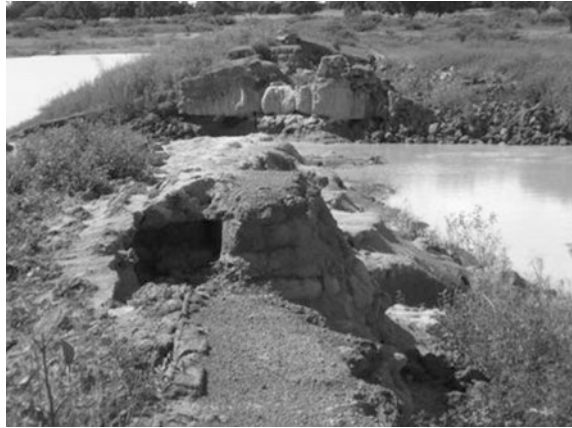
Fig. 4.3 Collapsed dyke at Tanghin. Photo by authors
