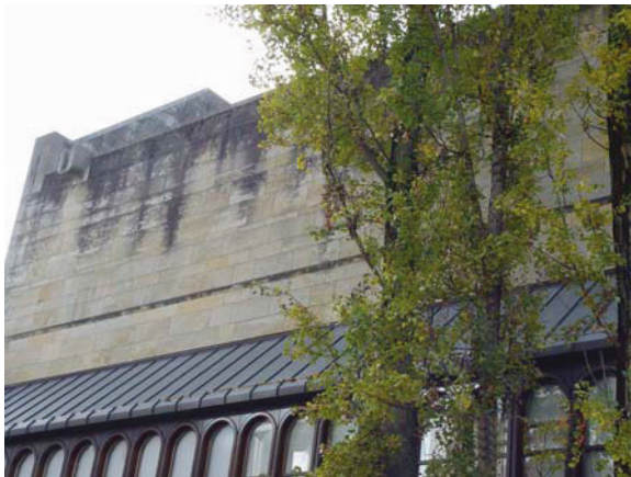
Fig. 5.6 Wall of the “Neue Pinakothek” München (Germany). Water runs down the sandstone plates and causes black biofilms also called “Tintenstrich-Flora” (ink-streak flora). Black soot or any air pollution particle can be excluded as the source of damage. The “Neue Pinakothek” was cleaned over a period of several years and a roof protection protruding only 3 cm horizontally from the rooftop was added contrary to the initial design of the architect according to whom the stones should directly meet the sky above
