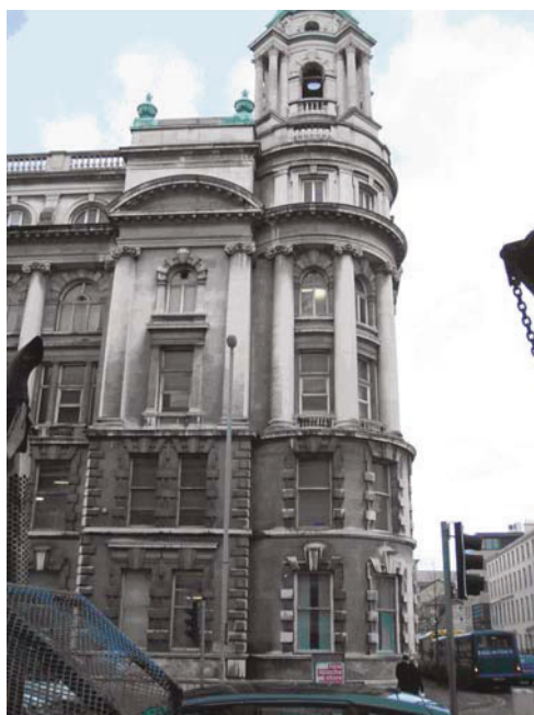
Fig. 4.1 Soiling on buildings in London, Belfast and Paris
