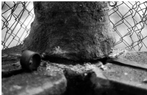
Fig. 8.20 Stone deterioration of the Black Tower in Ceske Budejovice by synergistic wind action
