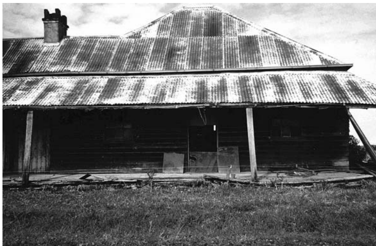
Fig. 3.1 Corroded roof of corrugated galvanised steel, the dark areas show the spread of rust
