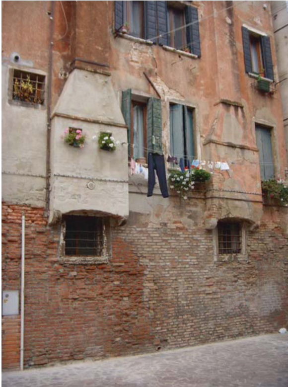
Fig. 6.27 Typical traditional Venetian popular house, Ramo primo agli Incurabili, Dorsoduro n° 436. (S = 96.80 m 2 : 100% render). Originally the entire brick surface was covered by the render which detaches at the basis of the walls due to capillary raisings and salt crystallisation (white efflorescences)
