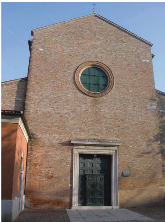
Fig. 6.26 Façade of the Sant'Agnese Church, Campo Sant'Agnese ( S = 158 \text{ m}^2 : 5% stone, 95% brick)
