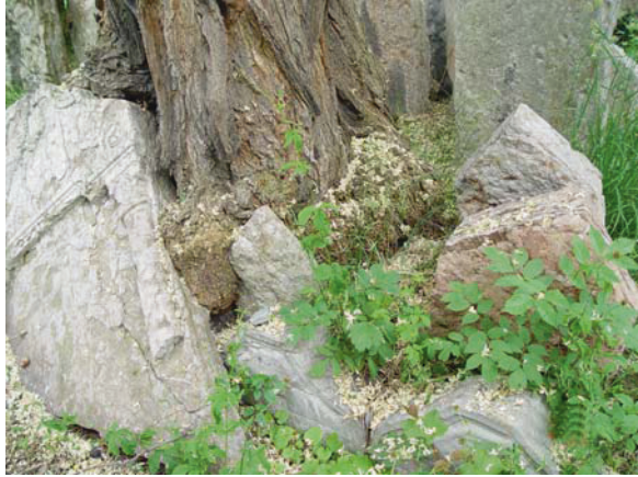
Fig. 5.3 Large tree roots deforming and crushing parts of one of the Temples in the Sanctuary of Angkor Vat (Cambodia). Mosses and smaller plants penetrate into crevices and cracks enlarging them and pushing the stones apart
