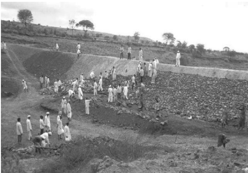
FIGURE 3.5 Stone pitching on the face of the earthen bund of a PT under construction. Photo from village Hiware Bazar, District: Nagar, Maharashtra State.
