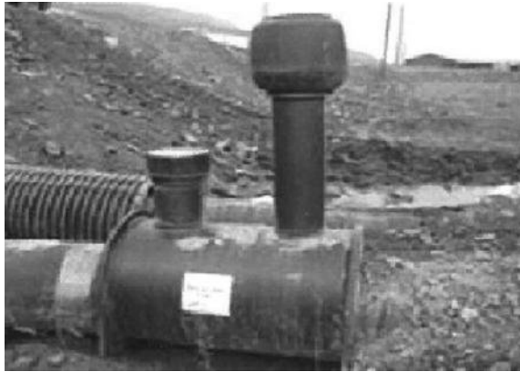
FIGURE 2.13 Sewer collection system; isolated pipes with heating cables. (From Longyearbyen Lokalstyre/Svalbard Samfunnsdrift, www.norvar.no/content/download/9434/104875 . Reprinted with permission from Ivar Undheim, Leader Longyearbyen Lokalstyre, http://www.lokalstyre.no/ )
