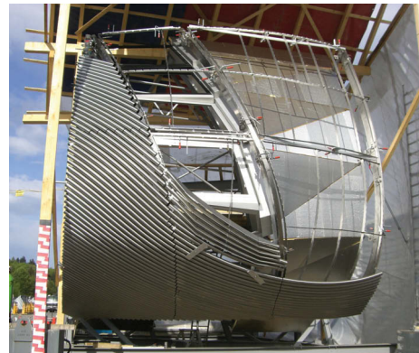
figs. 7–9 | Model, detailed rendering, and facade fabrication, King Abdulaziz Center for World Culture, by Snøhetta, Saudi Arabia, 2011
